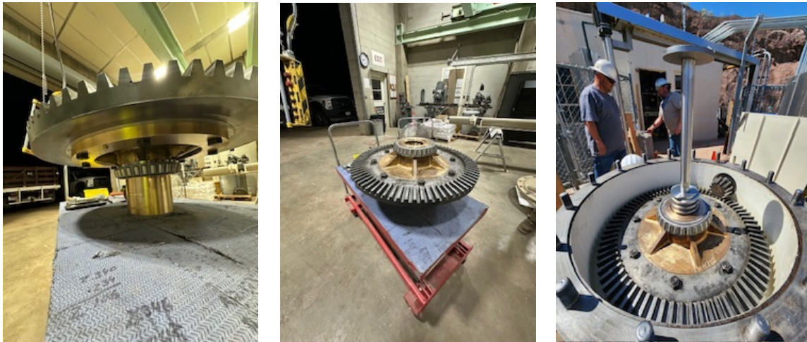
New bevel gear (left) and repaired actuator assembly (center and right) for gate at Copper Basin
