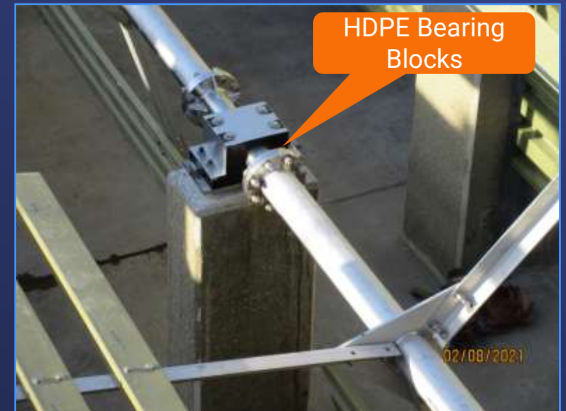
Flocculator Bearing Block
