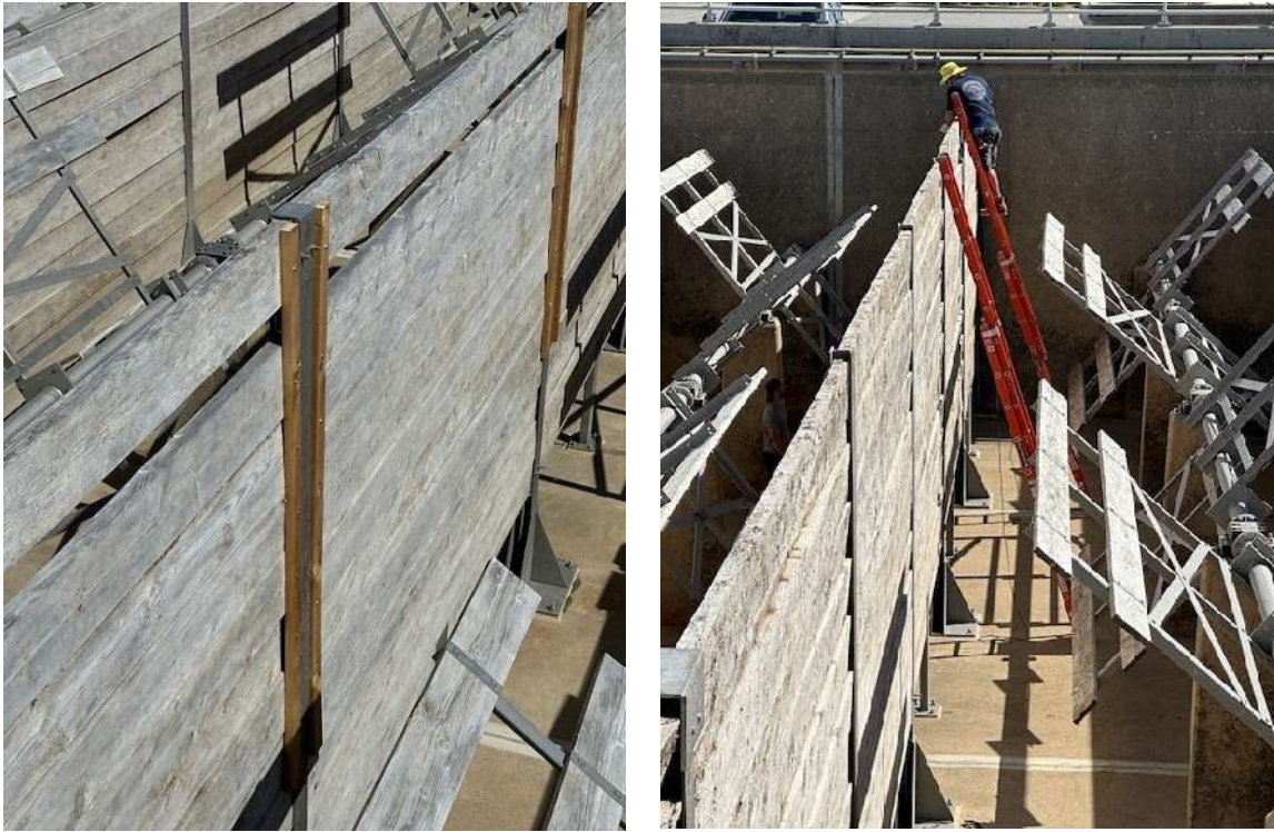
Staff securing baffle boards inside the sedimentation basin at the Diemer plant
