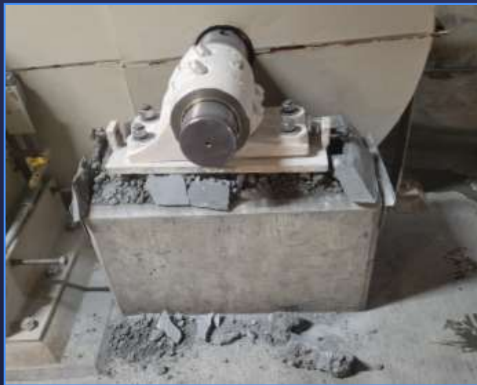
Anchorage failure at Basin 10
