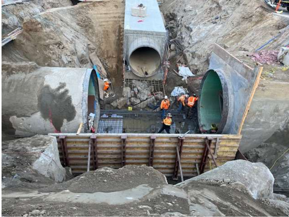
Wadsworth Pumping Plant Bypass— Constructing Forms For Encasement at the Tee Section
