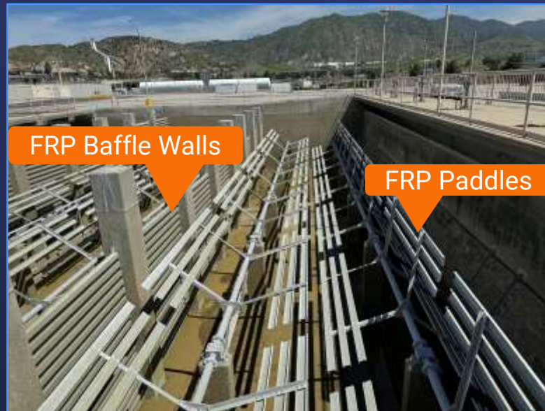
Flocculator shafts and paddle wheels
