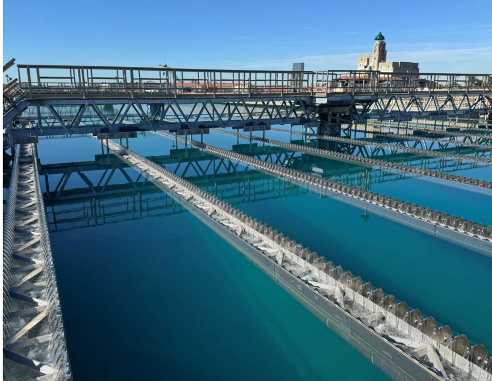
Weymouth Basins 5–8 and Filter Building No. 2 Rehabilitation— Filling Basin with Water for Initial Operational Testing
