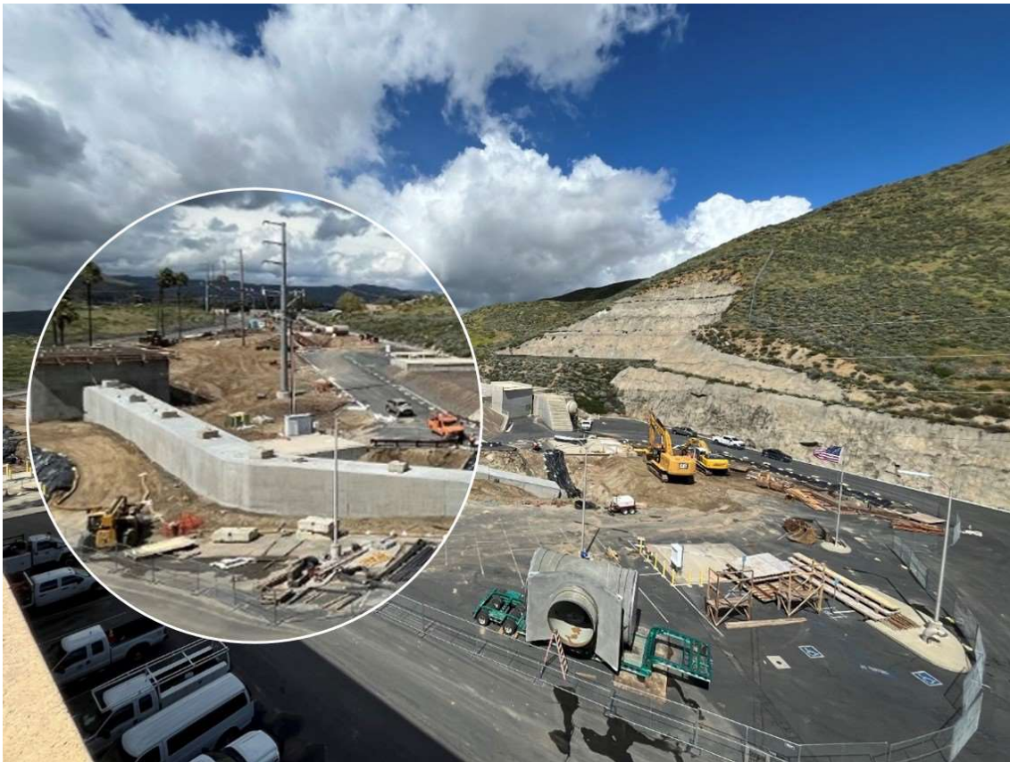
Newly constructed bypass encased in concrete to tie into existing piping at Wadsworth pumping plant at DVL
