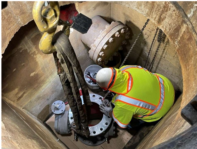
Staff installing a new lubricated plug valve on the Orange County Feeder
