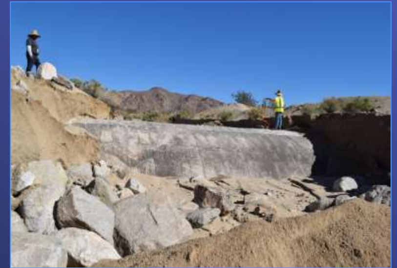
CRA Conduit Exposure from Storm (Oct. 2018)
