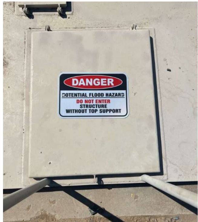
New warning sign to alert staff not to enter structure without top support
