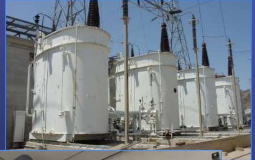
CRA Main Transformers
