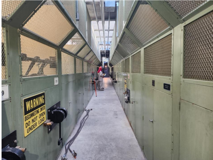
Staff performing switching in the 6.9kV switch house at Intake pumping plant
