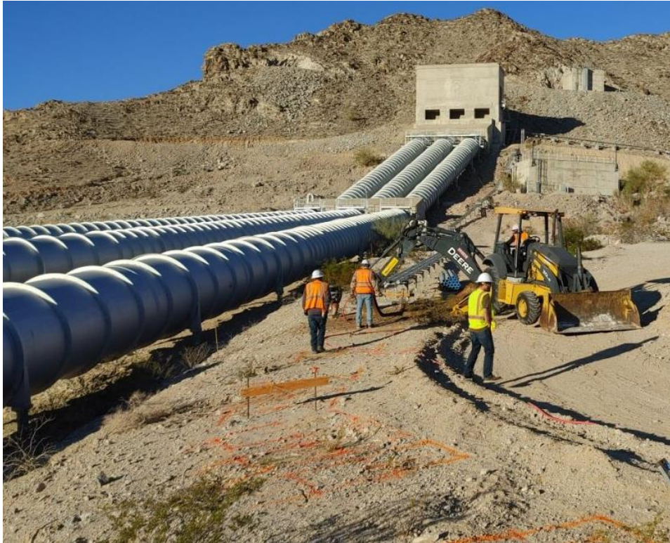
Domestic Water Treatment System Upgrades – Installing above ground conduit systems at Iron Mountain
