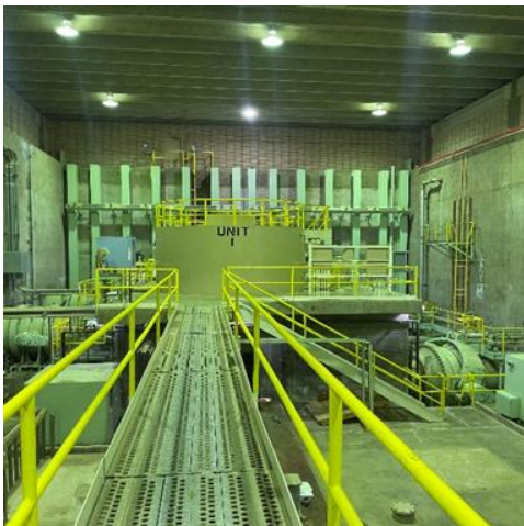
Foothill hydroelectric turbine Unit No. 1
