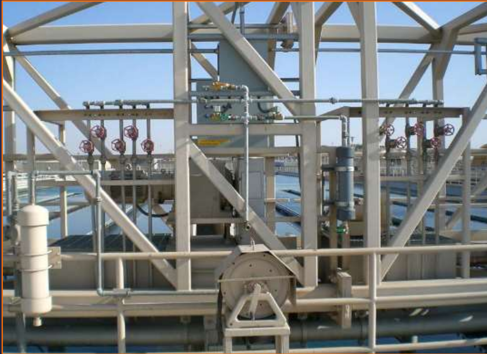
Existing Vacuum System
