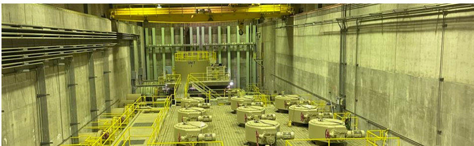
Foothill Pressure Control Structure
