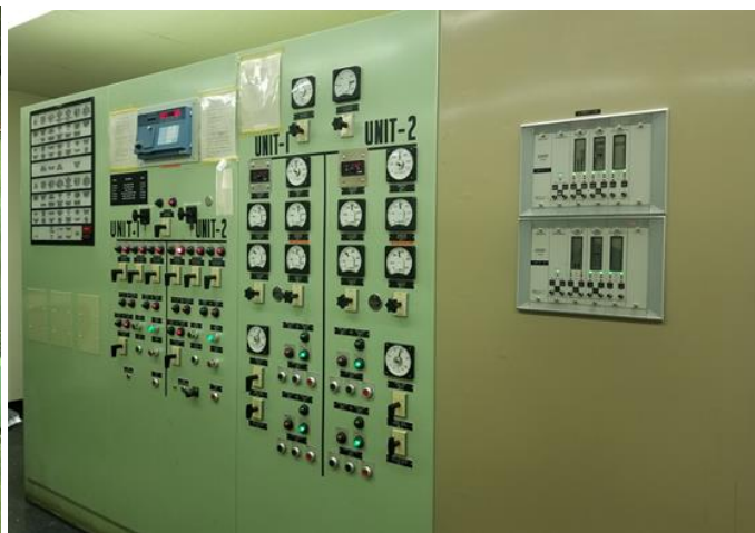
Foothill hydroelectric power plant control panel
