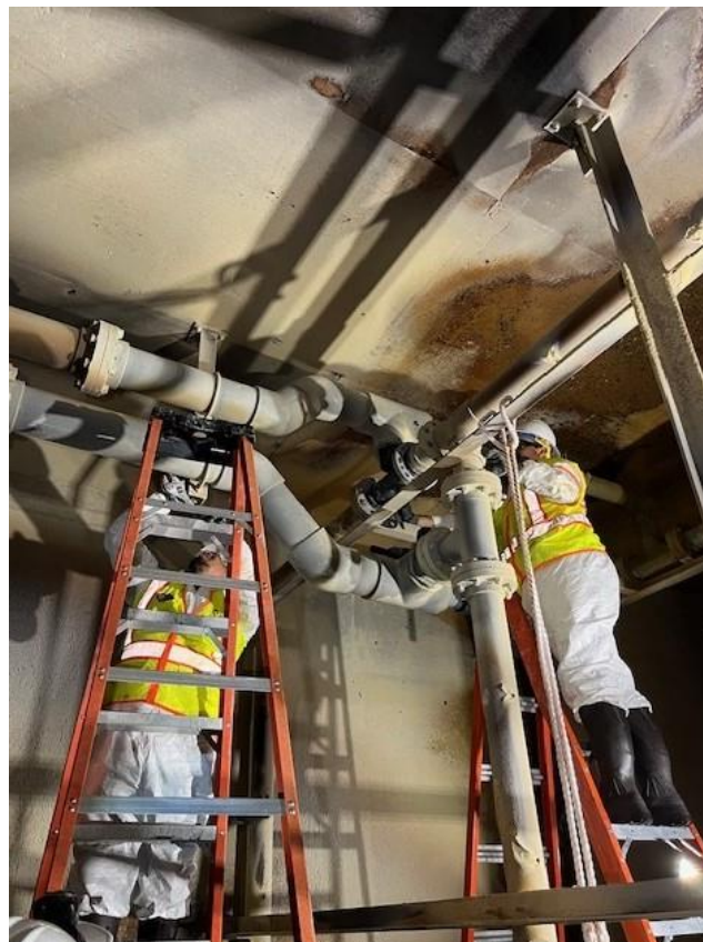
Staff repairing chlorine diffuser inside the combined filter effluent channel at the Diemer plant
