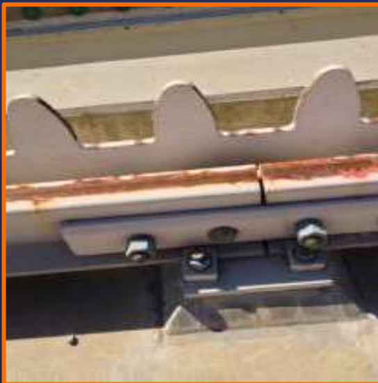
Gaps in rail
