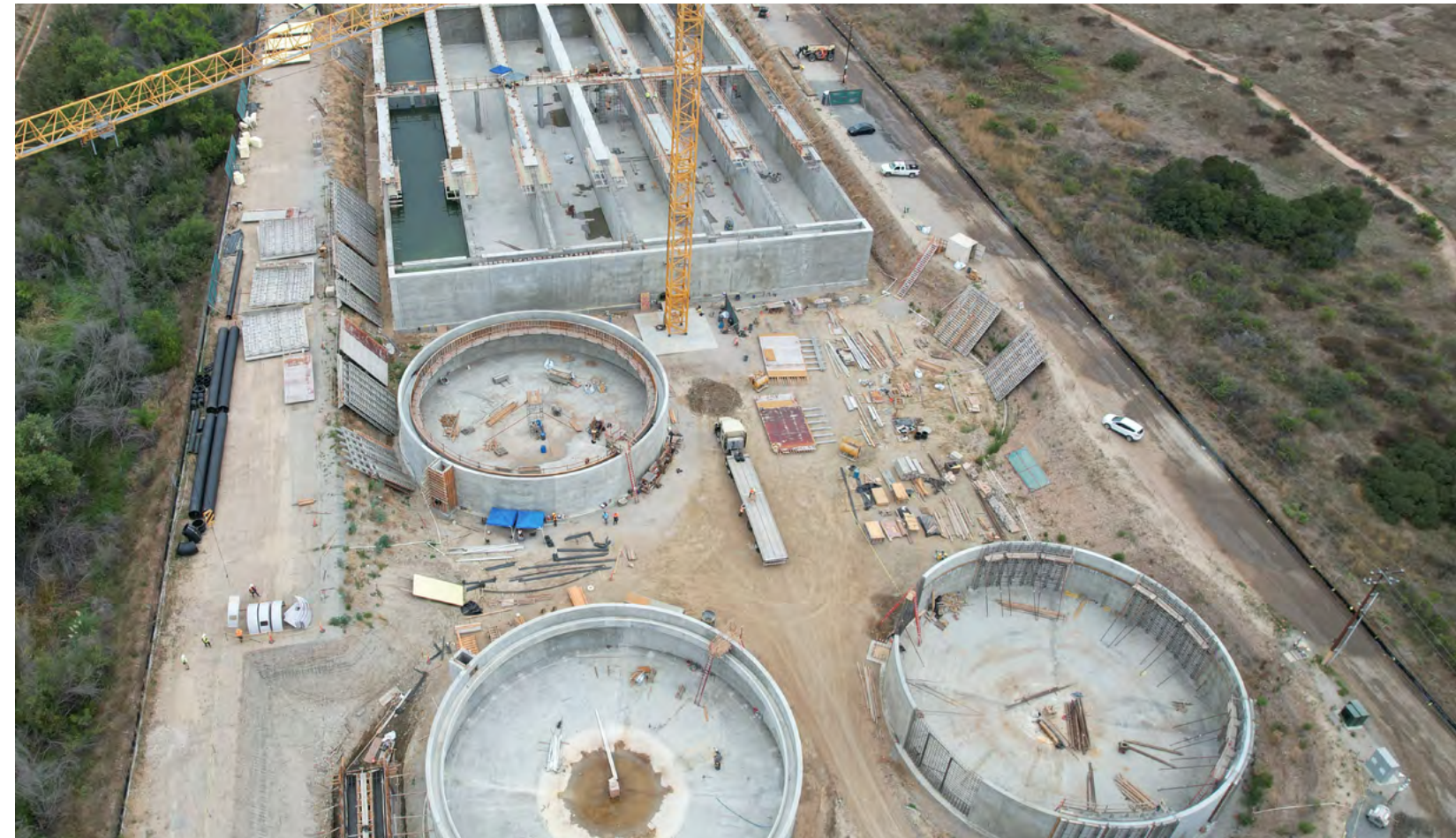
Construction of the East County Advanced Water Purification Project, a Local Resources Program project in the service area of the San Diego County Water Authority.
