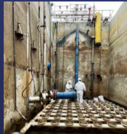
Critical Maintenance Needs
