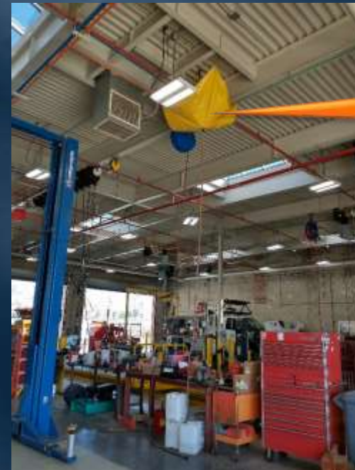
Temporary Rainwater Collection System
