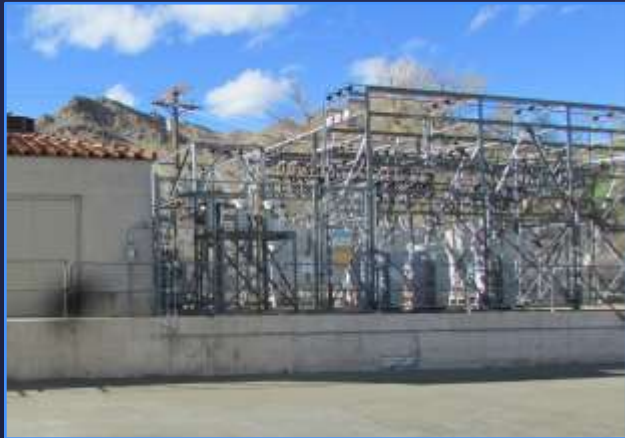
Station Light & Power Switchrack
