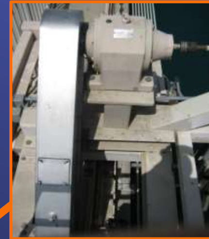
Motor drive at end of service life
