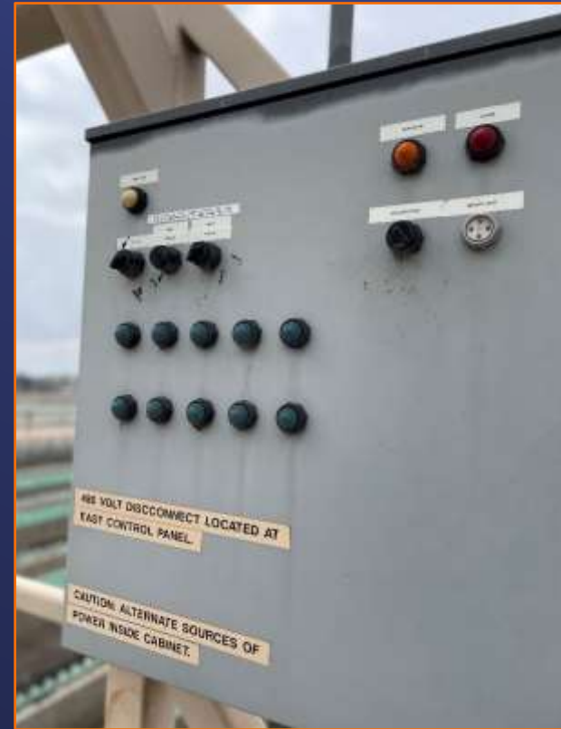
Existing Control Panel
