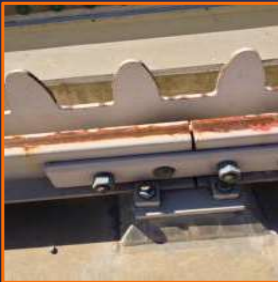
Gaps in rail
