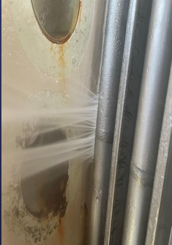
Initial leak on bellows joint
