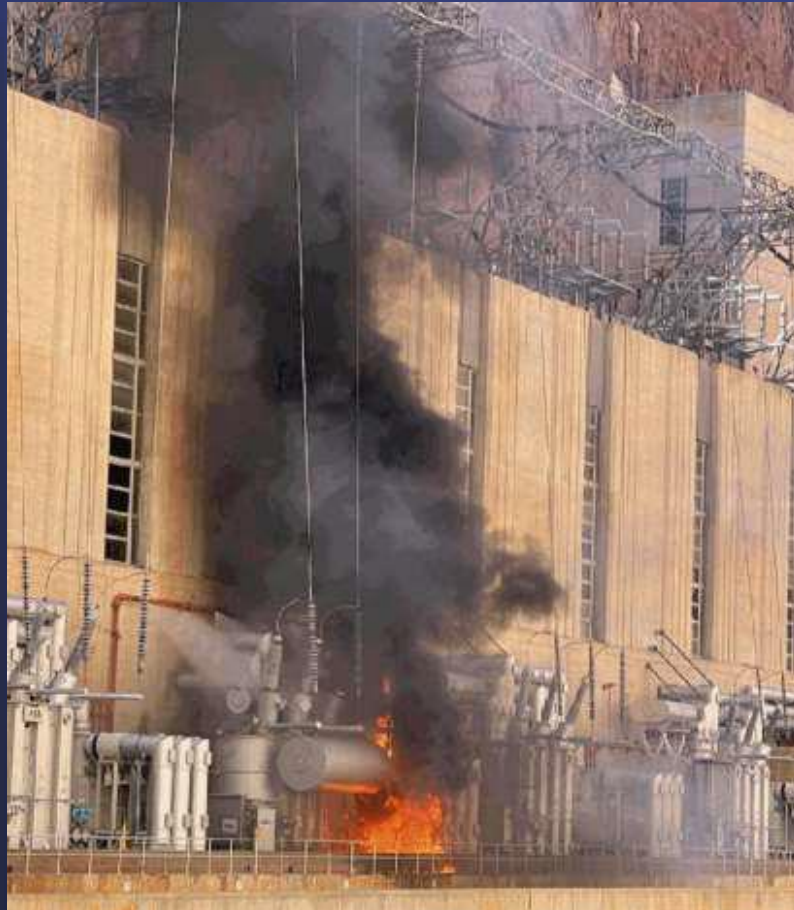
Transformer fire due to 230kV bushing failure
