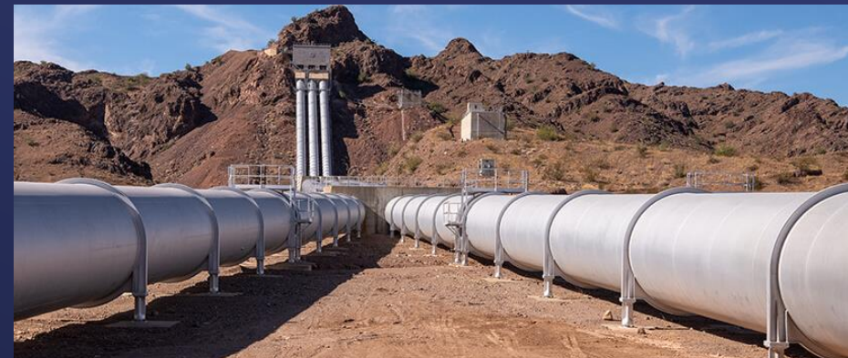
Gene Pumping Plant
