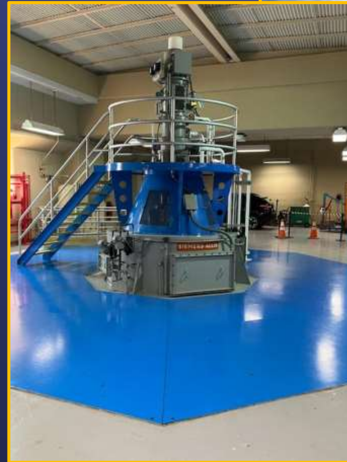
SWP Oso Pump Plant
