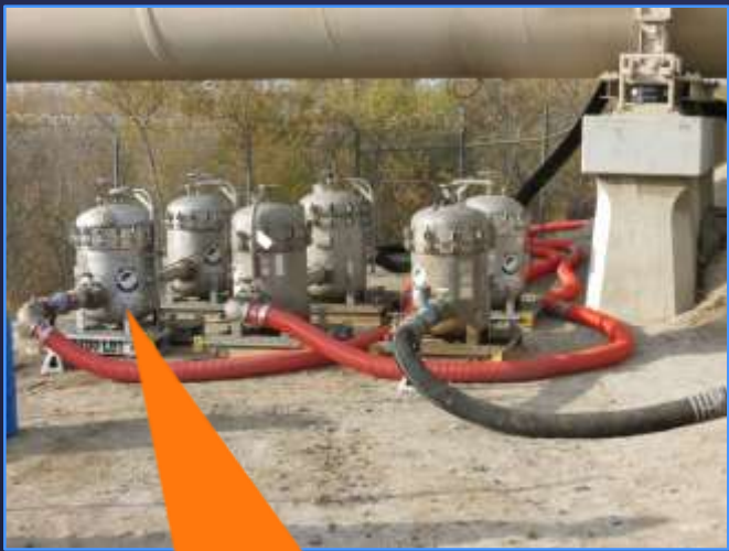
Quagga Filters for Dewatering
