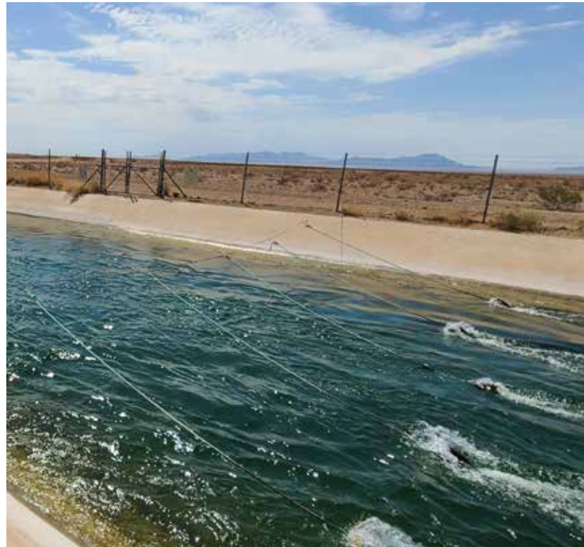
CRA operating at 8-pump flow
