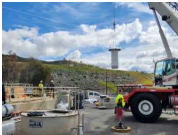
Staff lifting the bulkhead into position for installation at Red Mountain PCS
