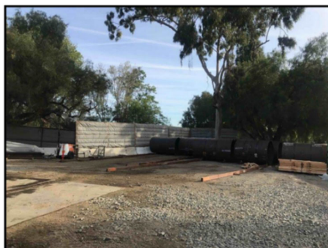
PCCP Second Lower Feeder Reach 3A Noise Barriers at Palos Verdes North Storage Area
