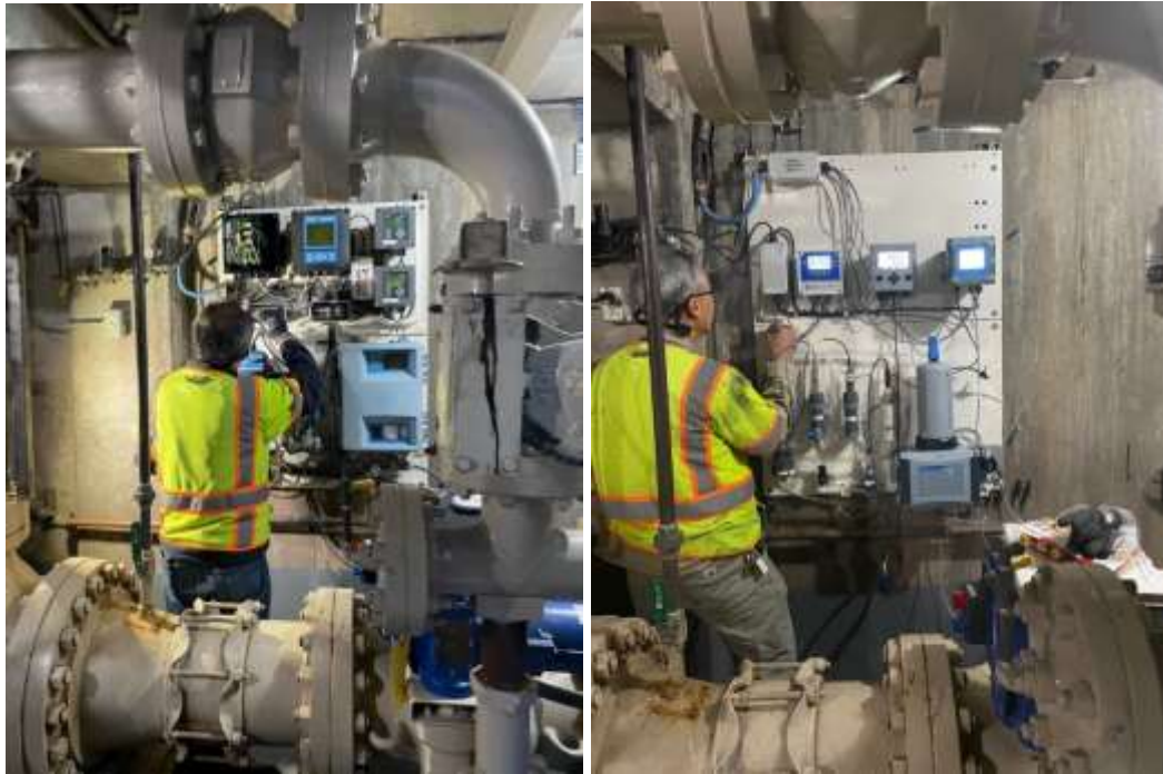
Staff removing old water quality panel (left) and installing new panel (right) at Beverly Hills PCS
