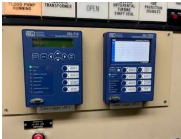
Newly installed data logger at Lake Mathews HEP
