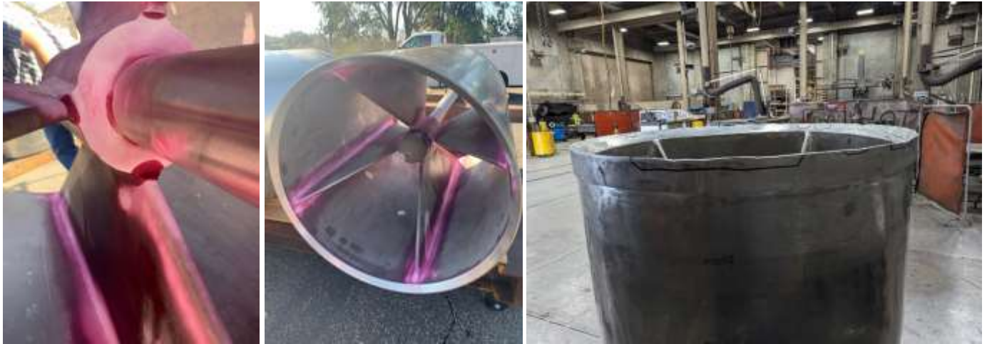
Dye penetrant test (left and center) and as-found damage on the sleeve valve gate (right) for Red Mountain PCS
