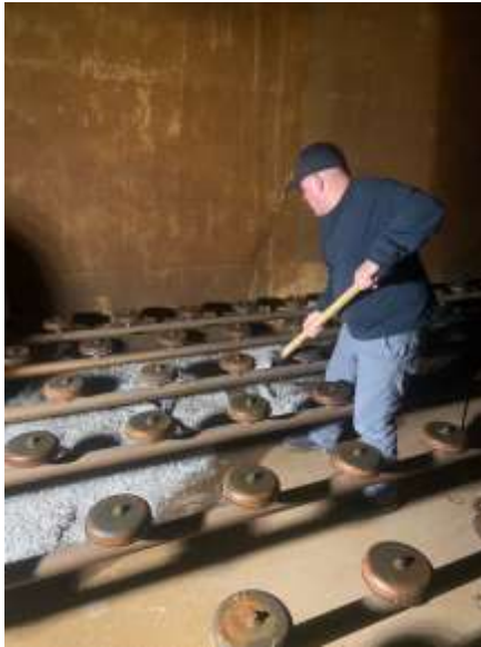
Staff removing quagga mussel shells around ozone diffusers inside Ozone Contactor #3 at the Diemer plant
