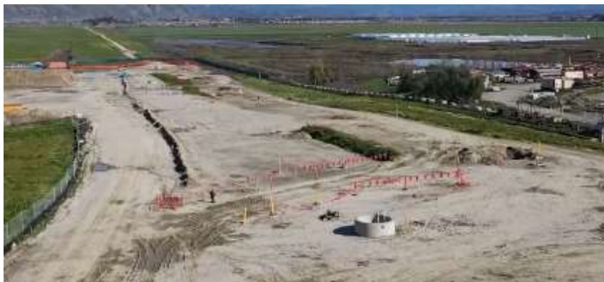
Casa Loma Siphon Seismic Upgrades—Casa Loma Siphon Barrel No. 1 site grading and restoration
