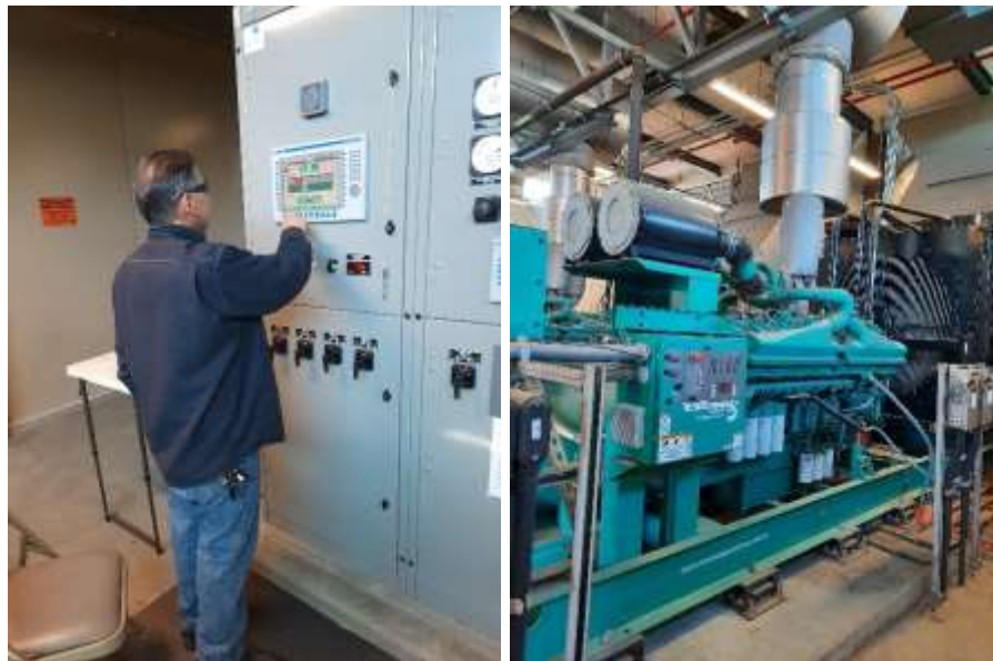
Staff performing testing of emergency generators (left) and associated equipment (right) at the Diemer plant
