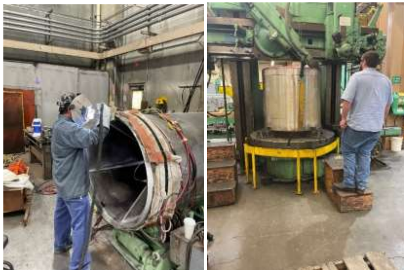
Staff weld-repairing valve gate (left) and machining of inner valve body (right) for Red Mountain PCS
