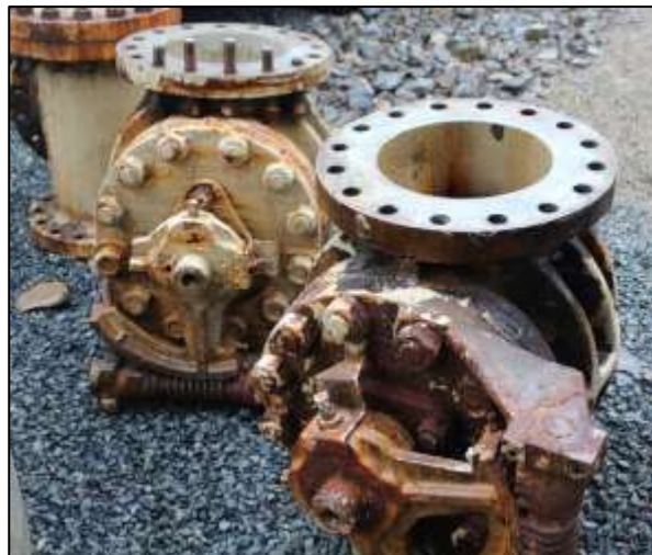
Corroded valves removed from the Santiago Lateral
