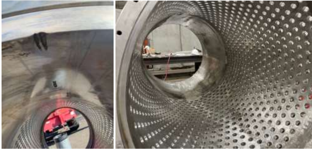
Damage discovered on outer valve body (left) and completed weld repairs (right) for Red Mountain PCS
