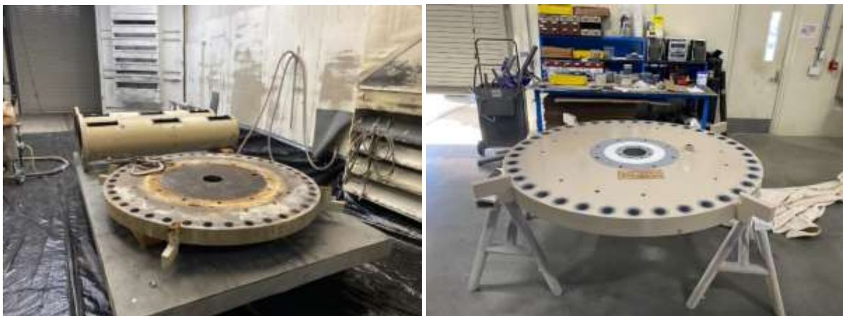
As-found sleeve valve cover (left) and completed valve cover (right) for Red Mountain PCS
