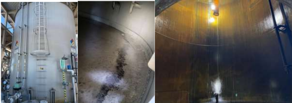
Outside of sulfuric acid tank (left); tank inside before cleaning (center); and inside tank after cleaning (right) at the Diemer plant
