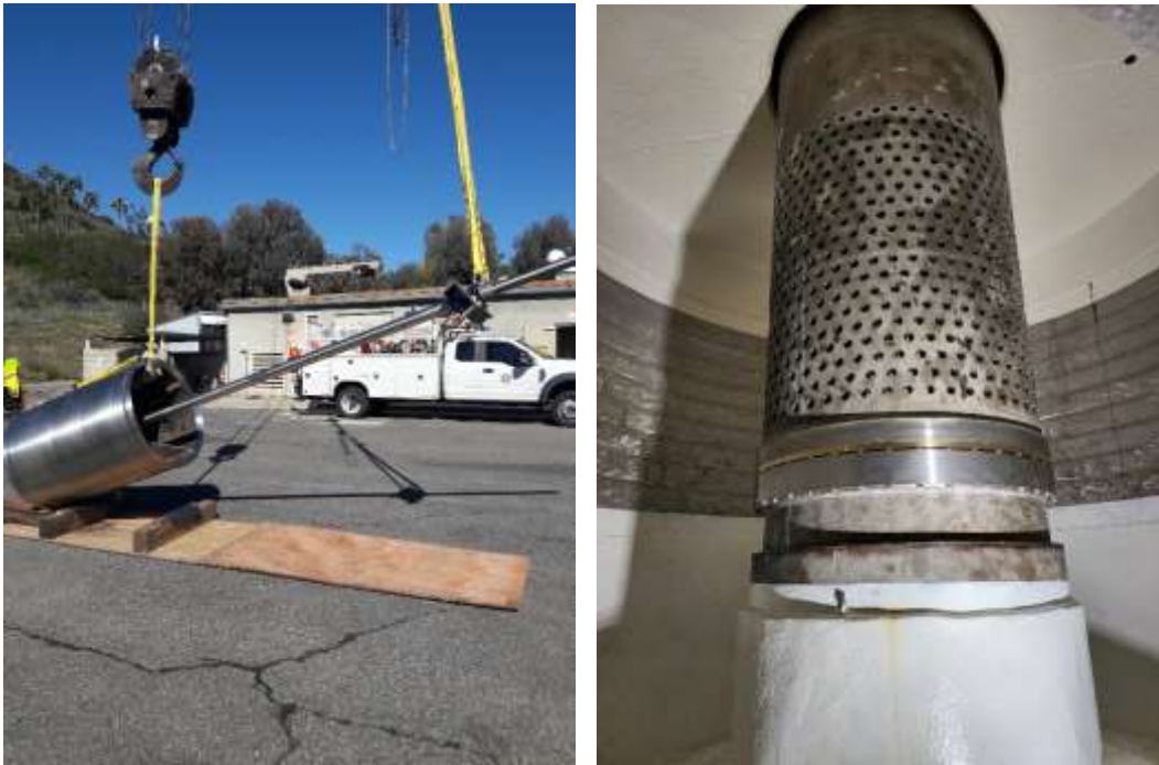
Rigging of valve gate (left) and sleeve valve installation (right) at Red Mountain PCS
