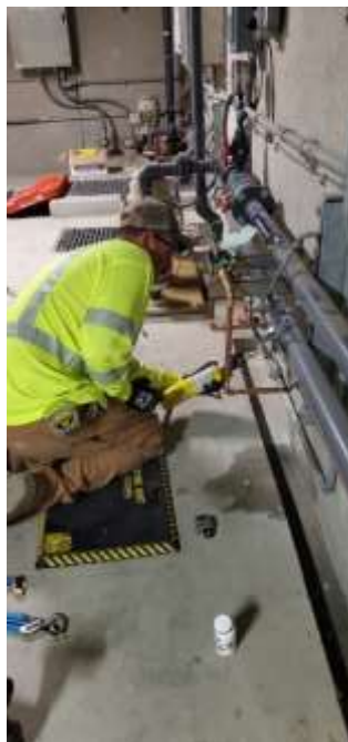
Staff installing backflow prevention device on sodium hypochlorite trench sump pump seal water supply line at the Skinner plant
