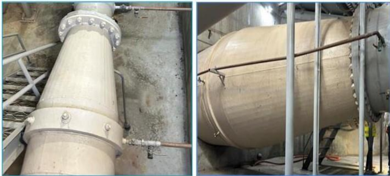
Existing LA-17A 24-inch venturi flowmeter (left) and existing 84-inch LA-17C venturi flowmeter in the City of Los Angeles
