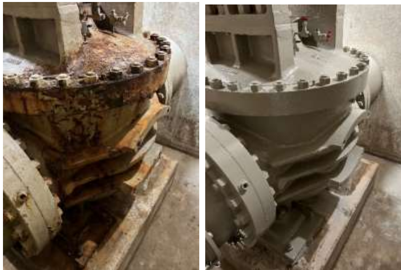
Before (left) and after (right) coating work on a plug valve at the PM-24 service connection
