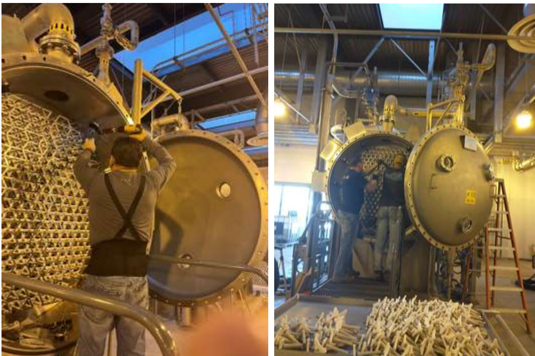
Staff installing new dielectric tubes and fuses in the ozone generators at the Jensen plant
