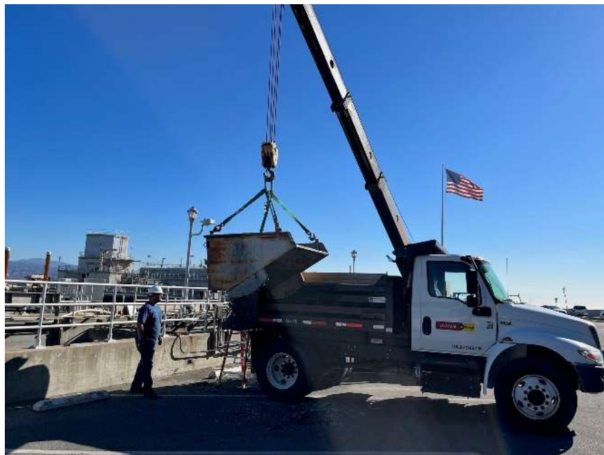
Staff removing solids and quagga mussel shells during maintenance of the basin influent channel at the Diemer plant
