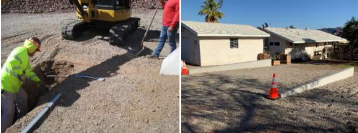
Staff excavating around buried utilities (left) and finished canopy footings (right) at a Desert facility residential structure
