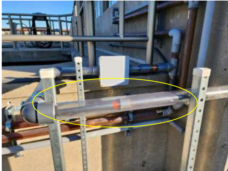
Double containment piping for the fluoride injection system at the Weymouth plant
