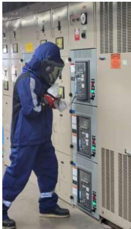
Staff safely racking out 4,160v breaker for maintenance at the Mills plant
