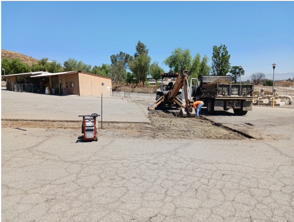
Preparing subgrade for paving over the newly installed sewer line near Lake Mathews Building 6
