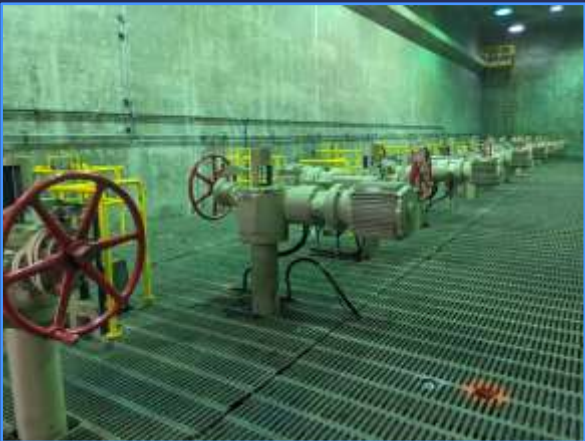
Venice Pressure Control Station
