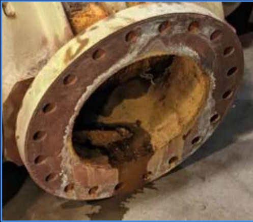
Existing Corroded Valve
