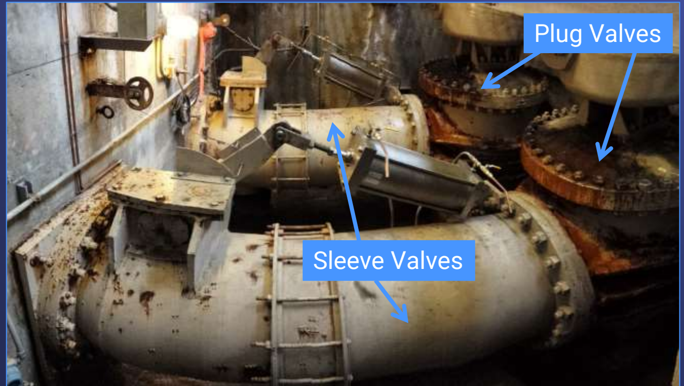
Existing valves at Hollywood Tunnel North Portal PCS
