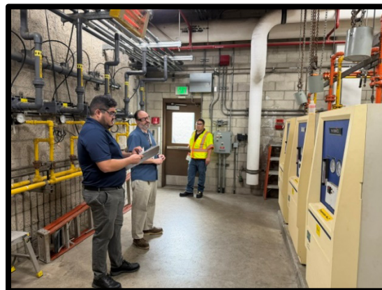
Triennial Safety Audit at Diemer Plant
