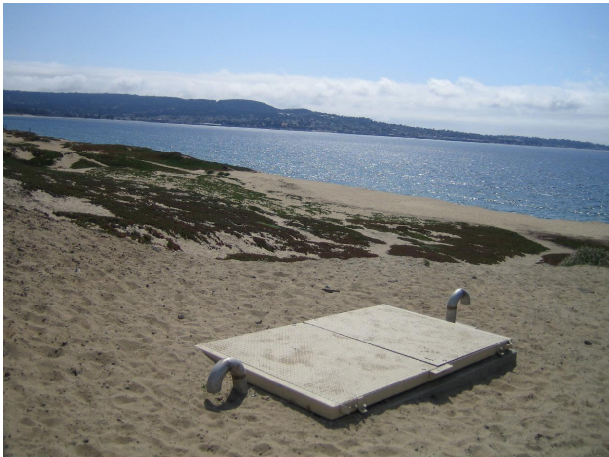
Figure 3.18 Vertical Beach Well at Sand City Desalination Plant
