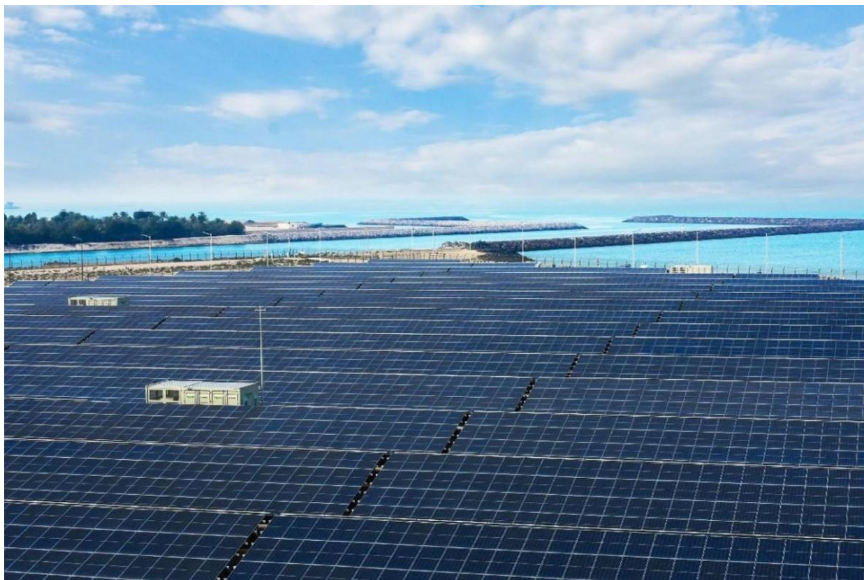
Figure 3.17 70-Megawatt Solar Farm Powering the Taweelah Desalination Plant (ACWA Power)
