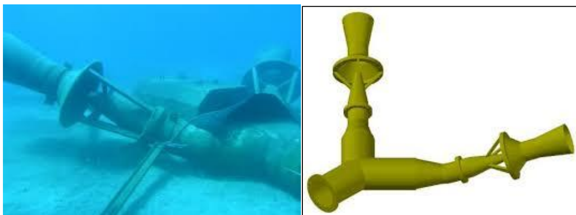
Figure 3.24 Venturi Diffusers Installed on Maspalomas II Brine Outfall (ECOS, Canary Islands, Spain)
