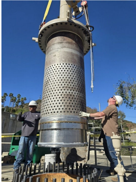
Staff installing a 42-in sleeve valve at the Red Mountain Pressure Control Structure
