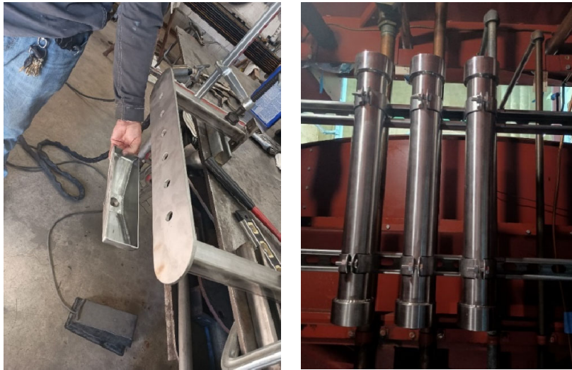
Lubrication oil sample tap bracket (left) and lubrication oil sample manifold (right)
