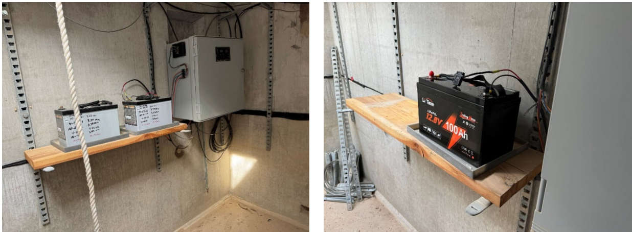
Old lead acid battery (left) and a new lithium battery installed (right)
