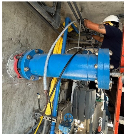
Installation of a new chemical line for the carbon dosing system at the PWSC Napolitano Center
