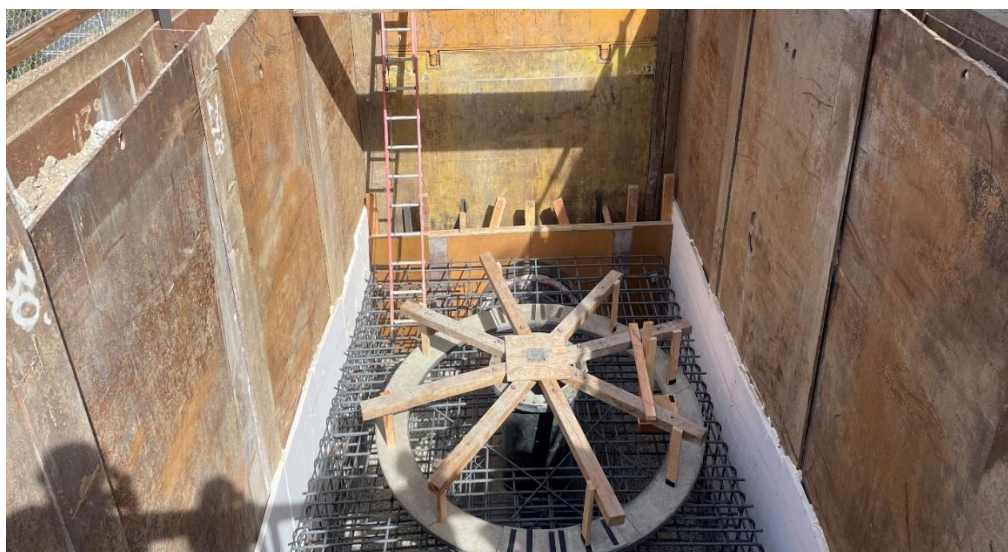
Stage 2 – concrete encasement forming and rebar installation for the pipe closure at an access site
