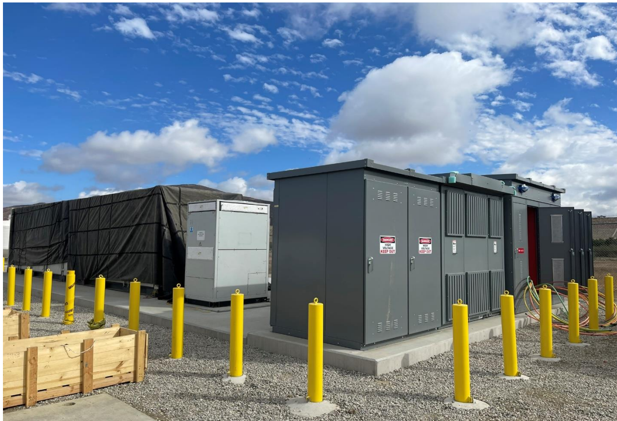
Battery Energy Storage System (BESS) enclosures at Skinner Plant
