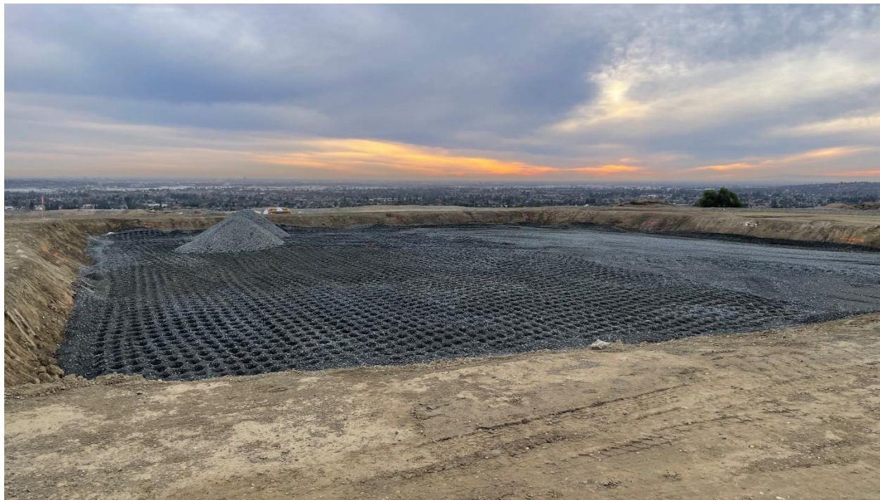
Helicopter landing pad at the Diemer plant – placing crushed aggregate for the pad subgrade
