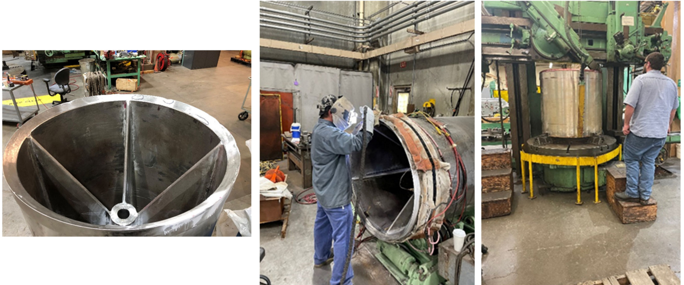
As-found valve gate (left), welding repairs of valve gate (middle) and machining of inner valve body (right)
