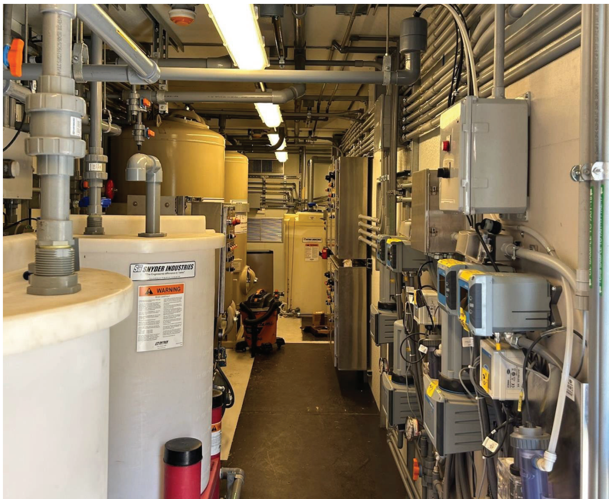
Spare unit water treatment skid at Intake Pumping Plant
