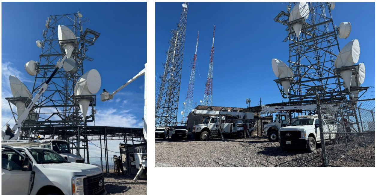
Las Vegas Junction communication site
