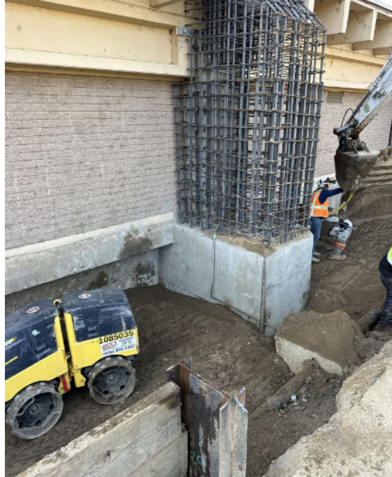
Foothill Hydroelectric Plant and Control Building Seismic Upgrade— Compaction around new building columns
