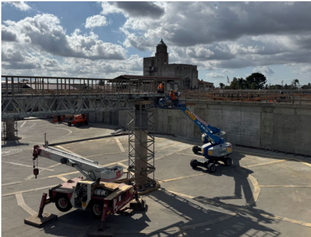
Weymouth Basins 5–8 and Filter Building No. 2 Rehabilitation— Installing the perimeter water line at Basin No. 6
