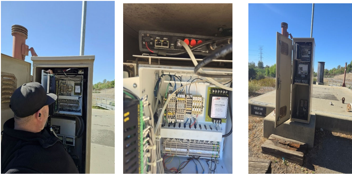
Staff completing radio upgrade (left), installed AMR radio and SCADA Pak (middle), and remote AMR service connection (right)
