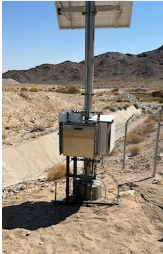
Water Level Sensor Installation — Completed installation of new level sensor enclosure on existing antenna pole
