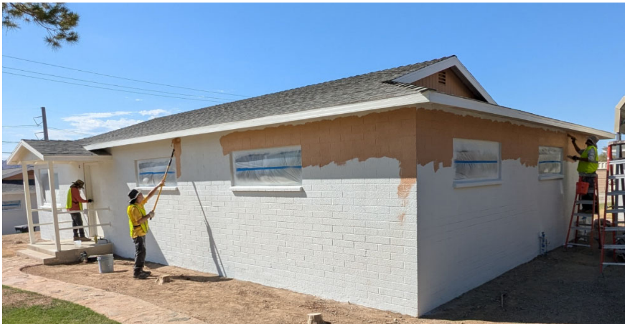
Colorado River Aqueduct District Housing Improvements— House Rehabilitation contractor applying first coat of Sierra tan paint
