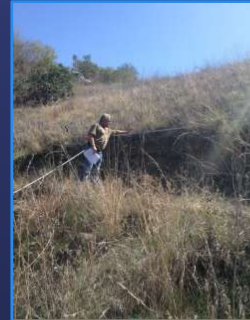
Slumped Toe Area of Basin No. 8 Slope
