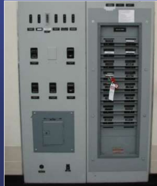
Typical Power Panel
