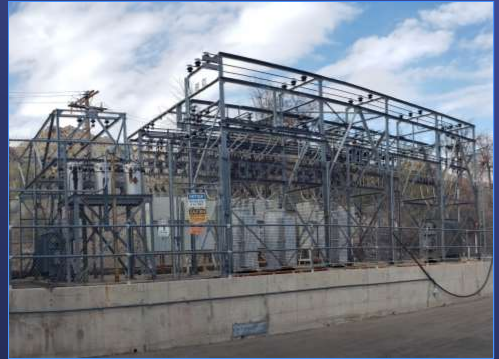
Existing 2.3 kV Switchrack (Iron Mtn.)
