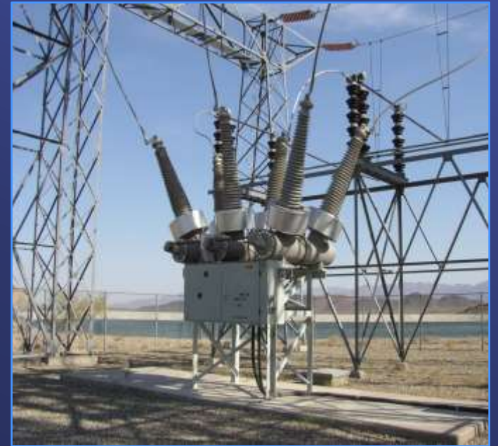
230 kV Circuit Breaker
