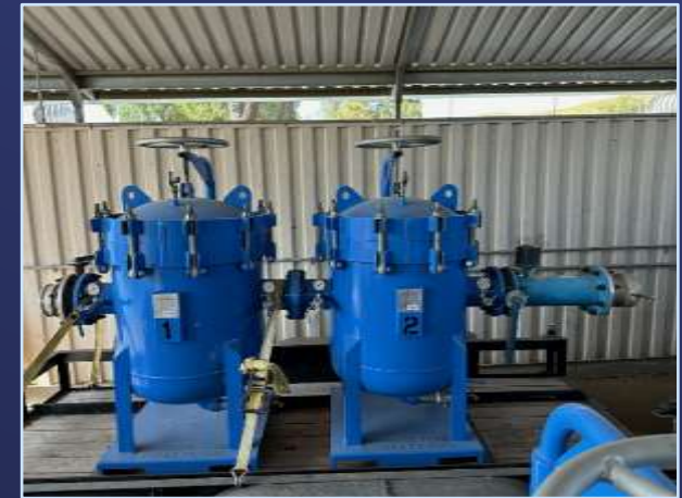
Filters for Raw Water Discharges
