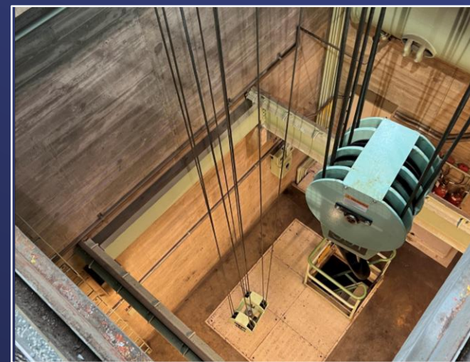
Hoists Below Motor Room Floor
