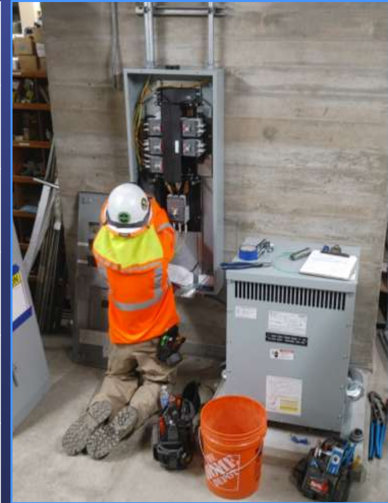
Electrical Panel at Intake Pumping Plant
