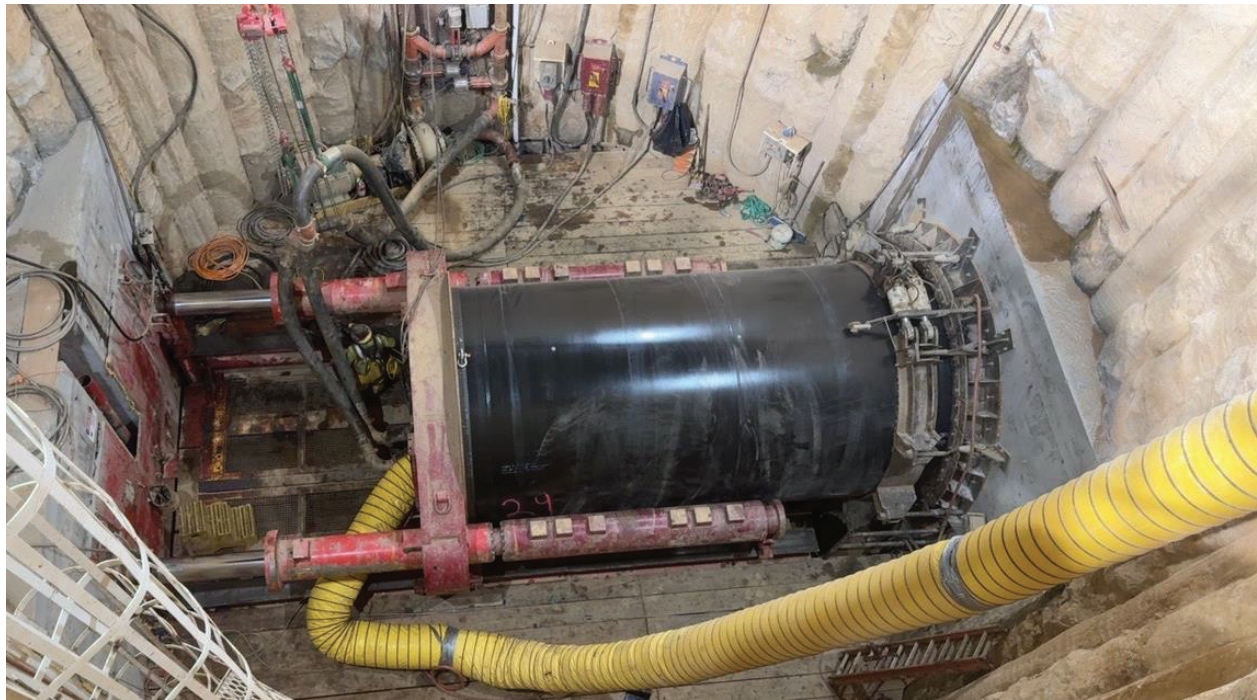
Secant pile shaft during installation of 120-inch diameter casing at Shaft No. 1 to the northern tie-in of Perris Valley Pipeline
