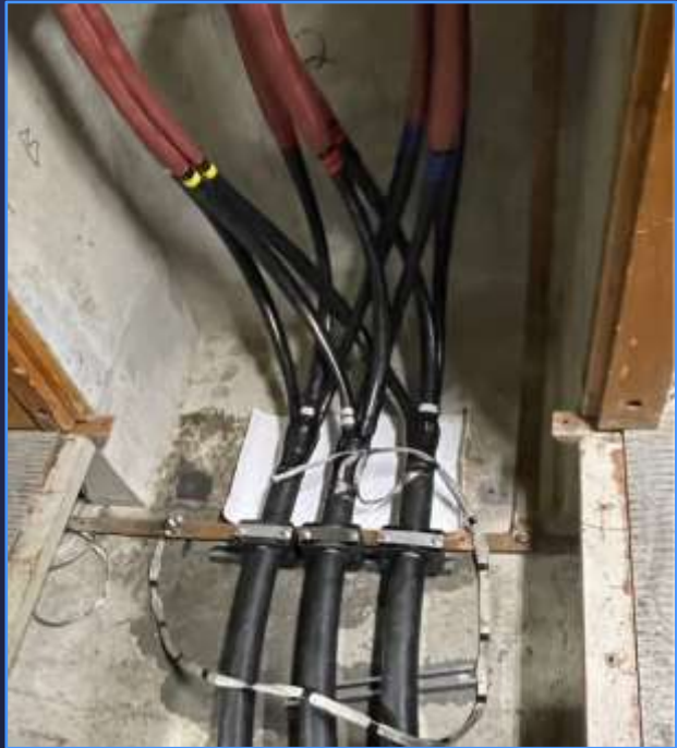
W.A. Chester LLC Terminated Cable
