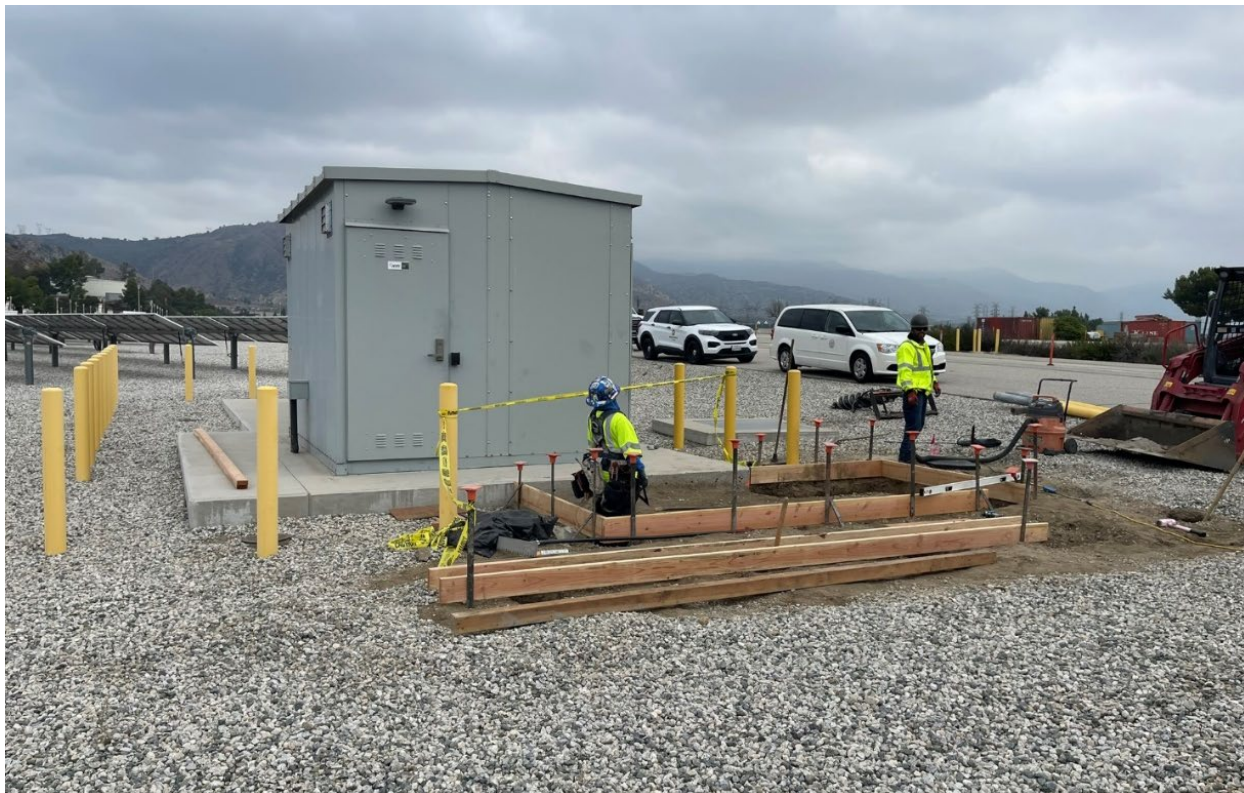
Constructing a protective relay panel cabinet foundation next to the solar facility at the Jensen plant
