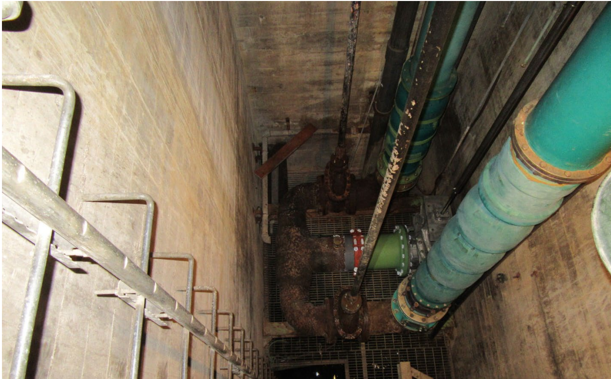
Existing sump system at Gene Pumping Plant
