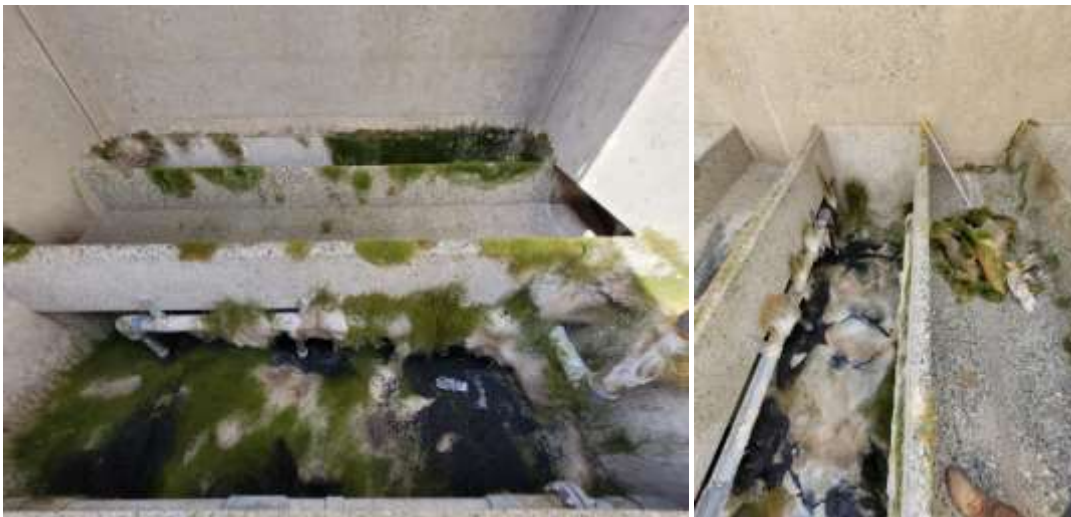
Filter and wash water trough before cleaning at the Jensen plant
