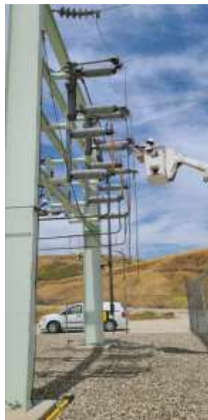
Staff performing switchyard maintenance at Foothill HEP
