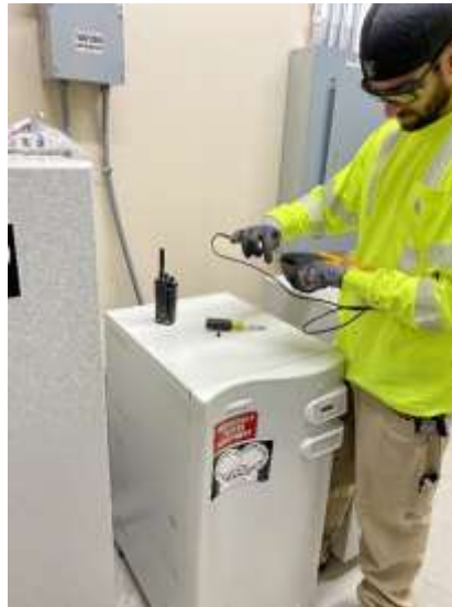
Staff testing UPS components in Building 4 at the Weymouth plant
