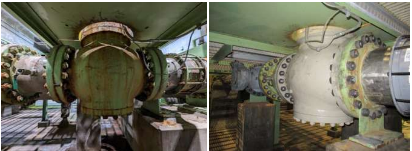
Leaking globe valve before (left) and after (right) refurbishment at Oak Street PCS
