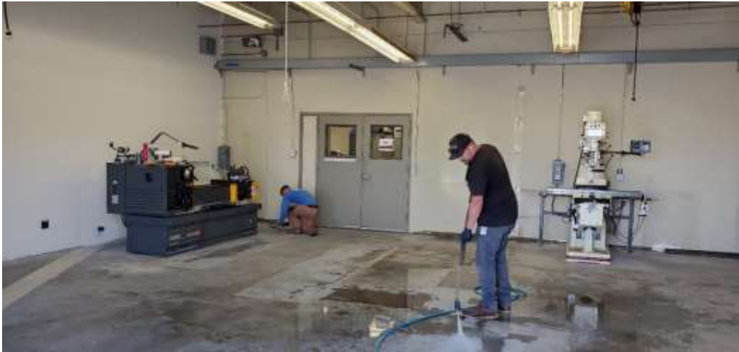
Staff pressure wash and prepare the workshop floor to receive epoxy coating at the Skinner plant
