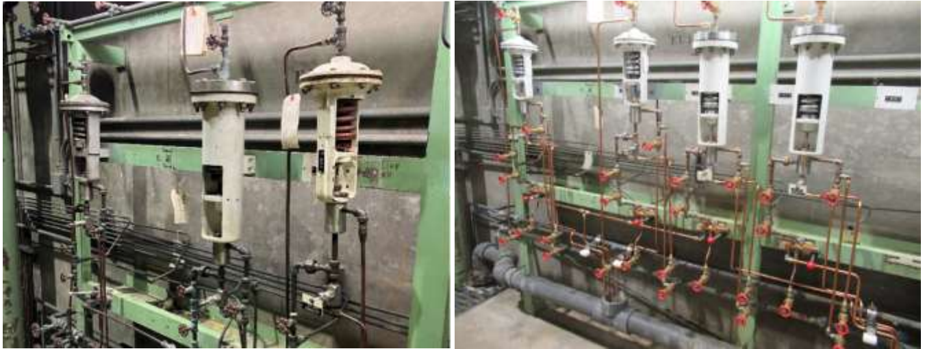
Before (left) and after (right) rehabilitation of the pilot rack at Oak Street PCS
