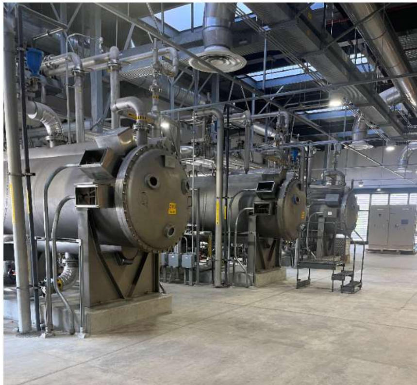
Jensen Ozone PSUs Replacement —Installed Generators 2 and 3 with High Voltage DC Cable
