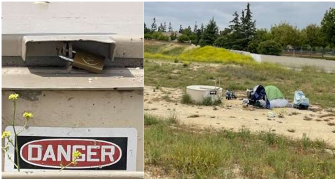
Security specialists and Western Region C&D staff partner to reinforce substructure lids along pipelines.
