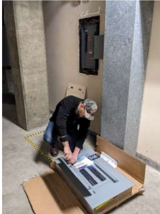
Staff preparing a new breaker panel for installation at the Diemer plant
