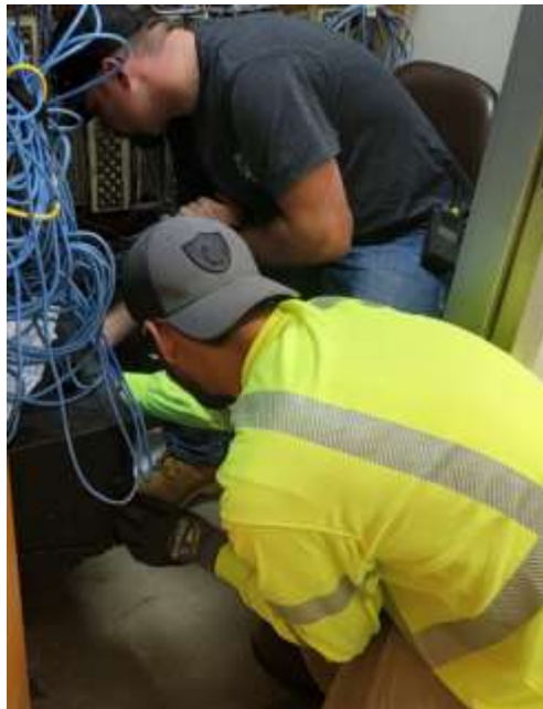
Staff diagnosing UPS in Building 40 at the Weymouth plant
