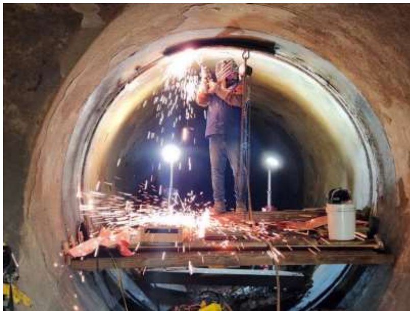
Staff torch cutting the remaining pieces of the large bulkhead installed at Perris PCS
