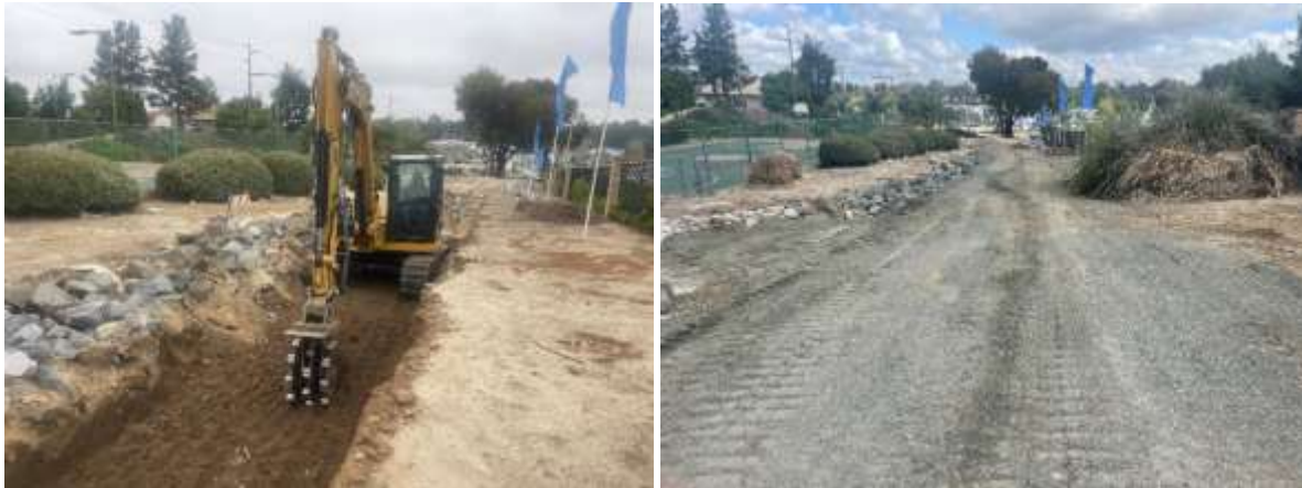
Staff using an excavator to compact fill material (left) and a completed section of road (right) along San Diego pipelines
