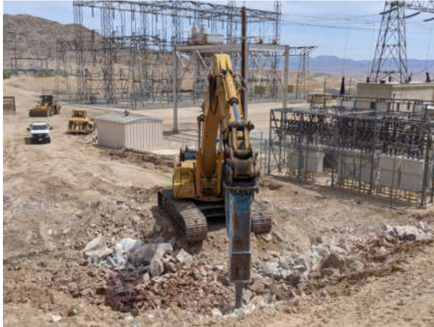
Staff hammering through rock and excavating at Iron Mountain pumping plant for the switch rack rehabilitation project
