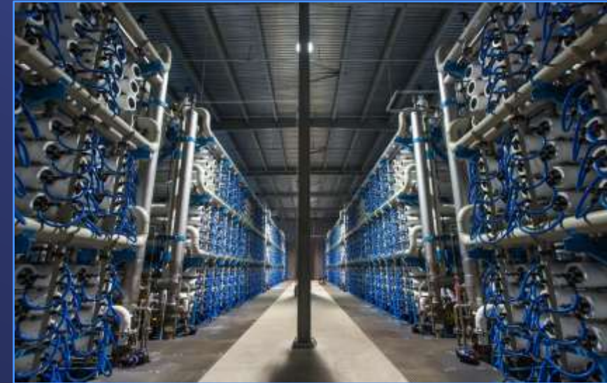
Claude "Bud" Lewis Carlsbad Desalination Plant
