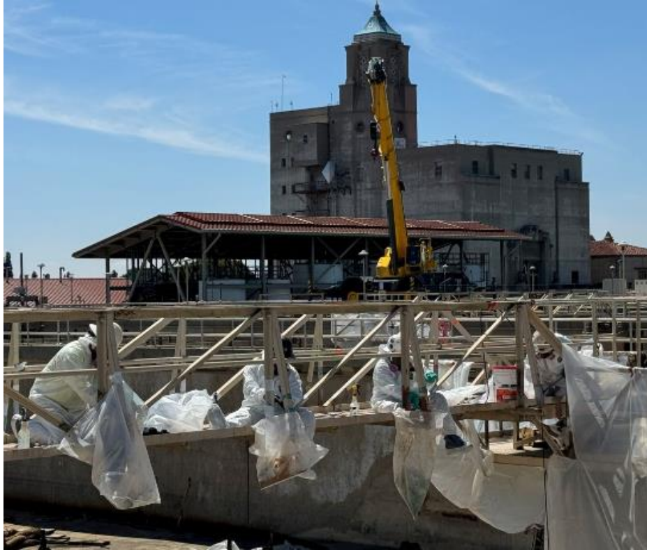
Weymouth Basins 5–8 and Filter Building No. 2 Rehabilitation Coating abatement at Basin 6 clarifier bridges
