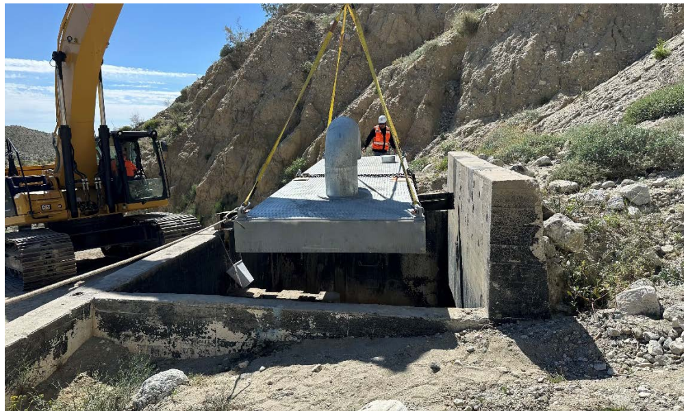
Transition Structure Cover Installation at Site 23 east of Hinds Pumping Plant near Desert Hot Springs
