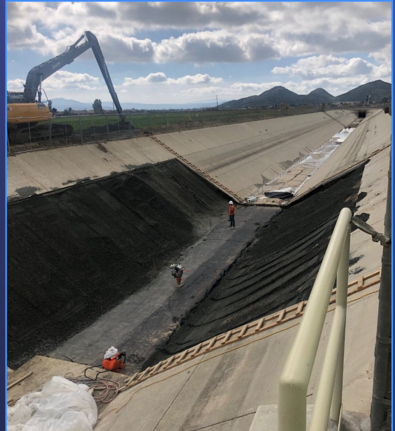
Contractor compacting aggregate base material along side slopes of San Diego Canal
