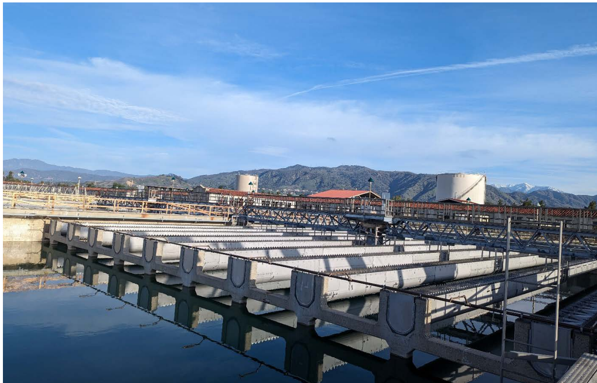
New stainless-steel launders in Basin No. 8
