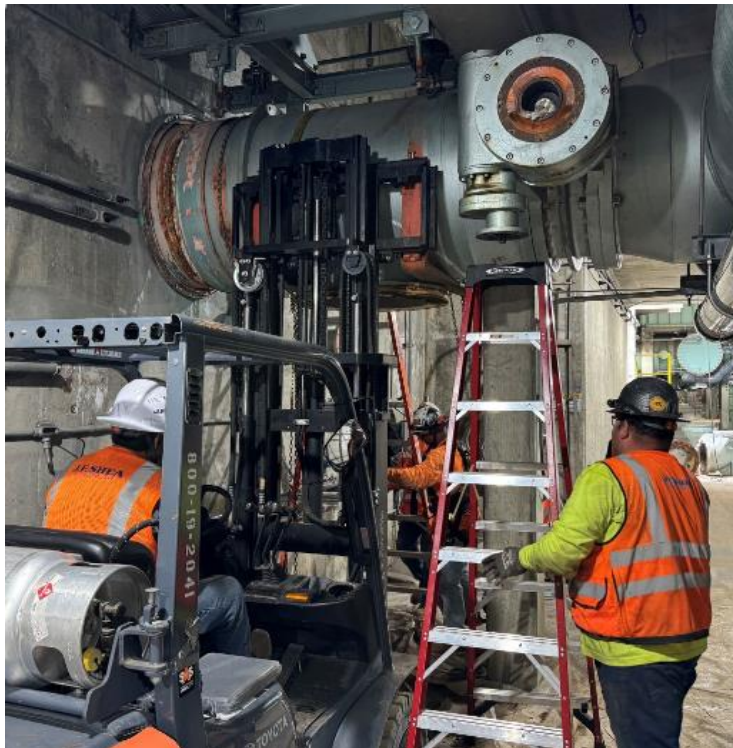
Weymouth Basins 5–8 and Filter Building No. 2 Rehabilitation Dismantling backwash piping at filter gallery for installation of new 30-inch backwash valve
