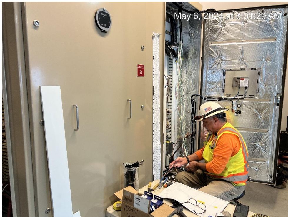
Termination of Power Supply Control Wires
