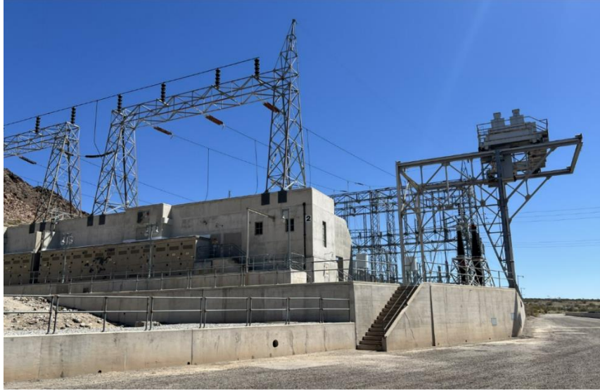
Hinds Pumping Plant Switch House
