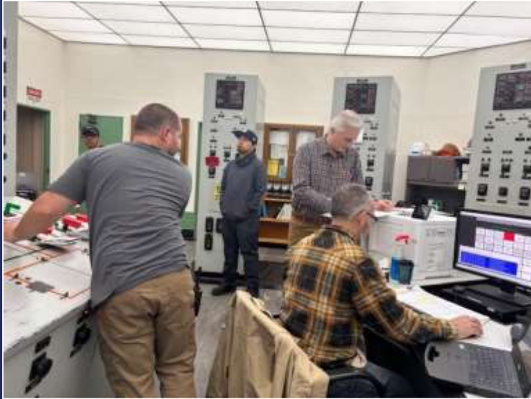
Gene PP transformer annunciator panel installation
