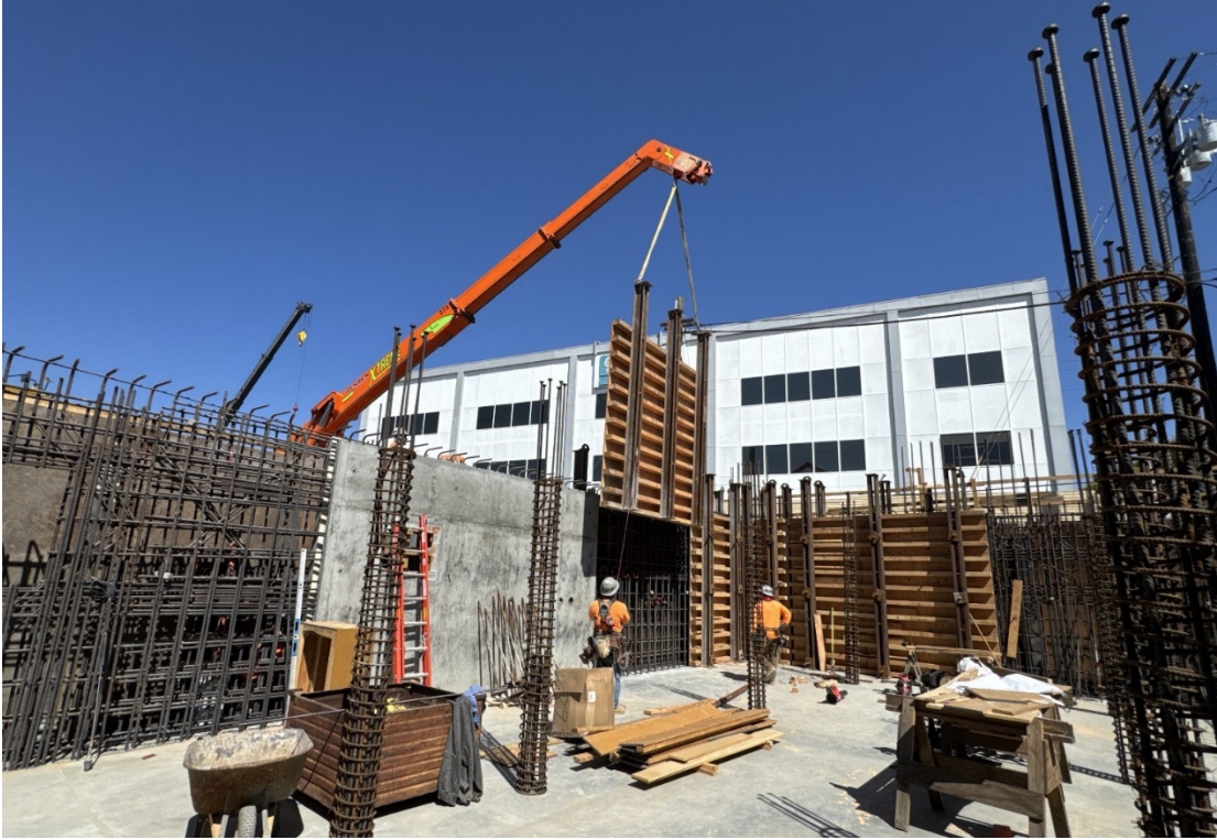
Sepulveda Feeder Pump Stations – Installation of Basement Wall Forms in Electrical Building
