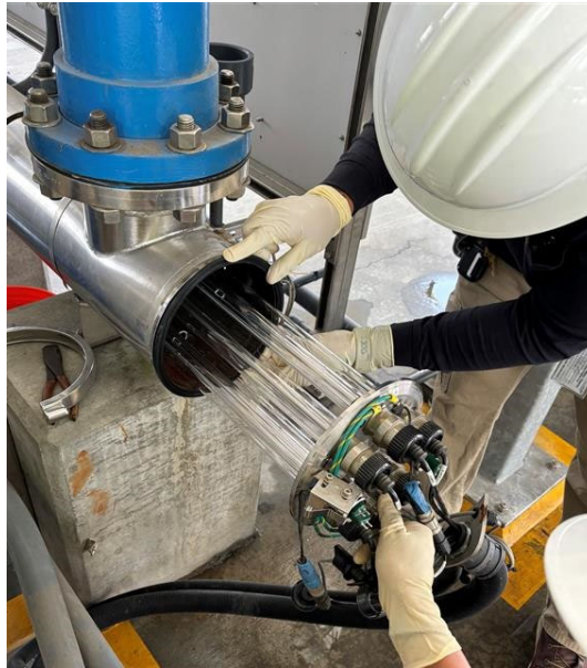
Staff replacing UV lamps for the advanced oxidation system at the PWSC NIC demonstration plant
