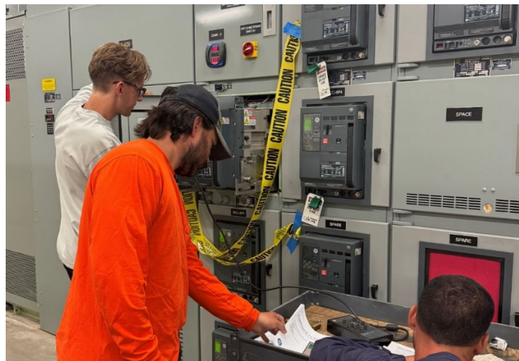
Staff testing a de-energized circuit breaker at the Skinner plant
