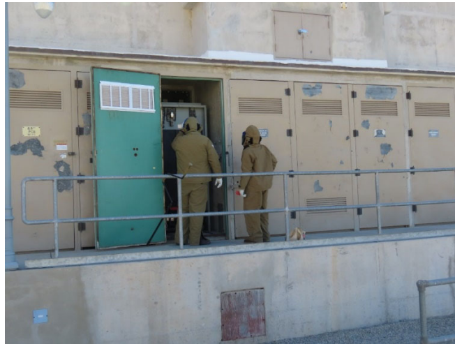
Staff racking out a 6.9kV circuit breaker at Hinds pumping plant
