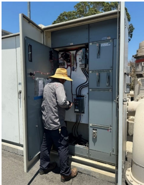
Staff installing electrical soft starters for Lake Skinner Outlet Tower chlorine pumps
