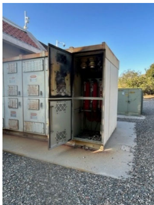
Failed surge arrester on incoming power line
