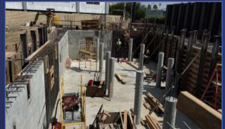
Sepulveda Feeder Pump Stations – Venice PS
