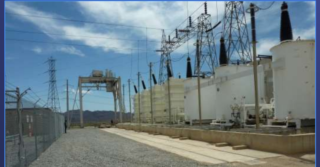
CRA Main Transformers
