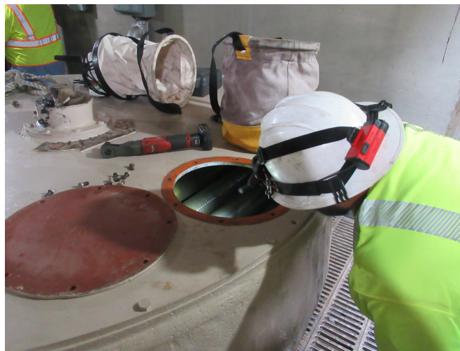
Staff inspecting the interior of a valve during routine preventive maintenance
