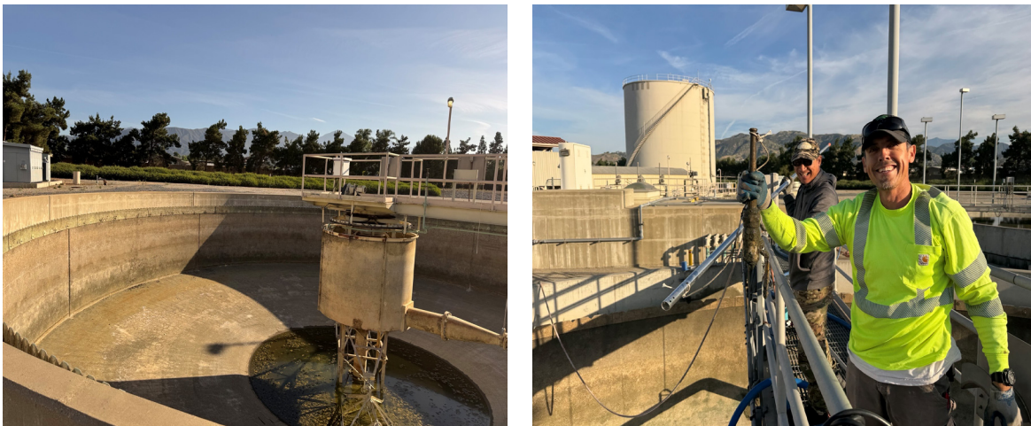
Thickener after cleaning (left) and staff cleaning thickeners (right) at Weymouth plant
