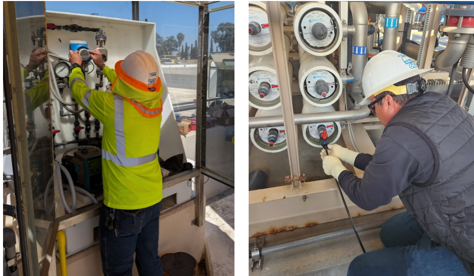
Repairing the MicroC carbon chemical injection system (left) and inspecting a reverse osmosis element (right) at the PWSC demonstration plant
