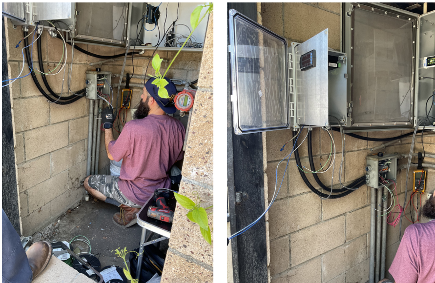
Staff installing new wiring for flow-capturing device (left) and new flow-capturing device panel (right) for solids monitoring at Weymouth plant
