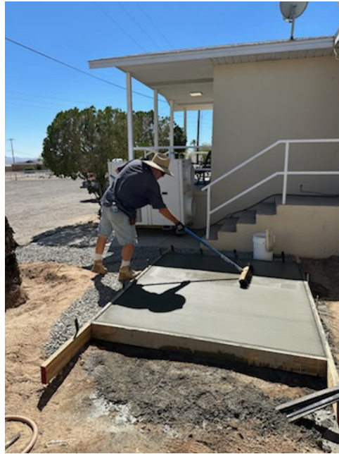
Staff building a concrete pad for new HVAC unit installation at the Iron Mountain dorm
