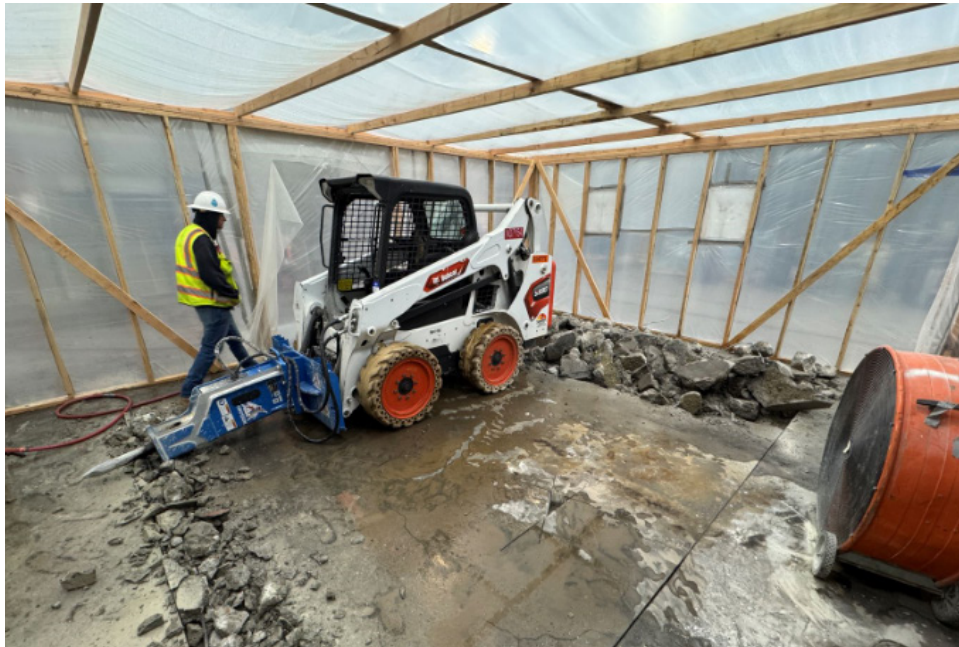
La Verne Shops Improvements —Slab Demolition for Vertical Band Saw Foundation at the La Verne Fabrication Shop
