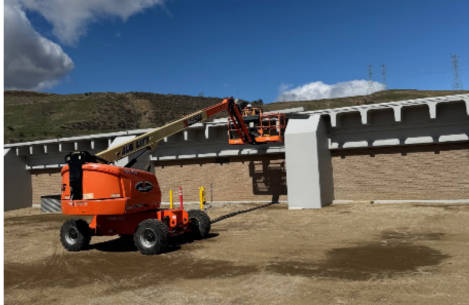
Foothill Hydroelectric Plant and Control Building Seismic Upgrade — Installing Painted Gutters onto the Building
