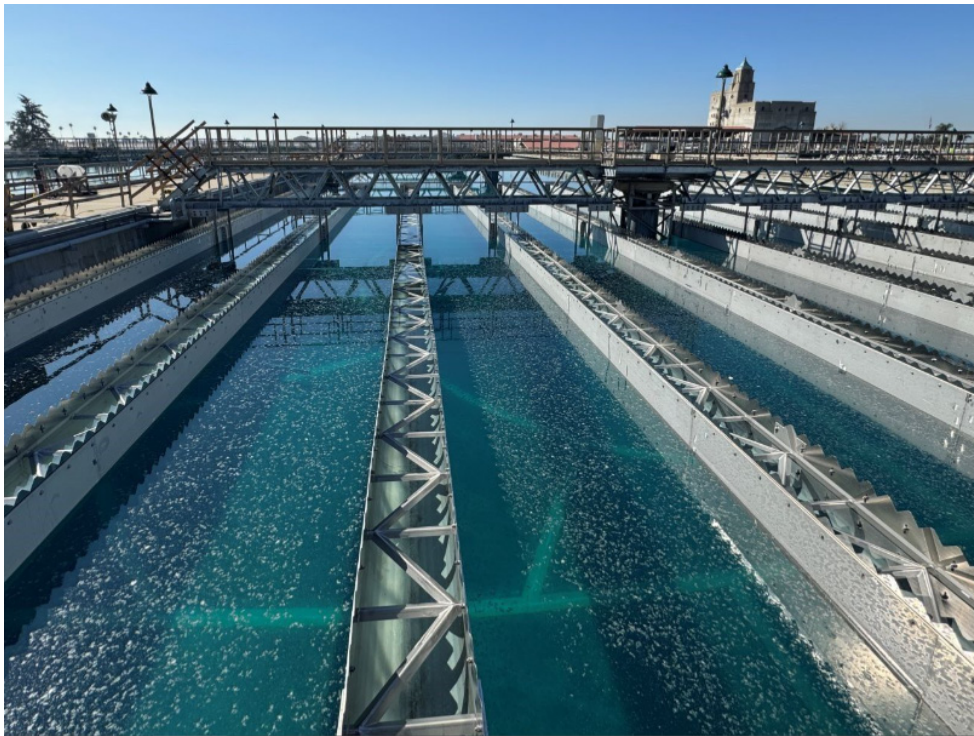
Weymouth Basins 5–8 and Filter Building No. 2 Rehabilitation —Filling Basin 6 for Performance Testing
