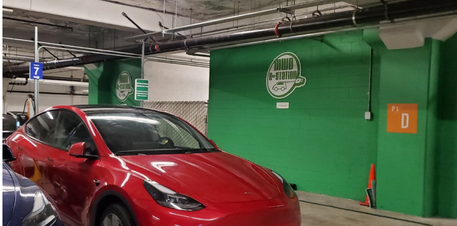
Existing EV charging station at Headquarters
