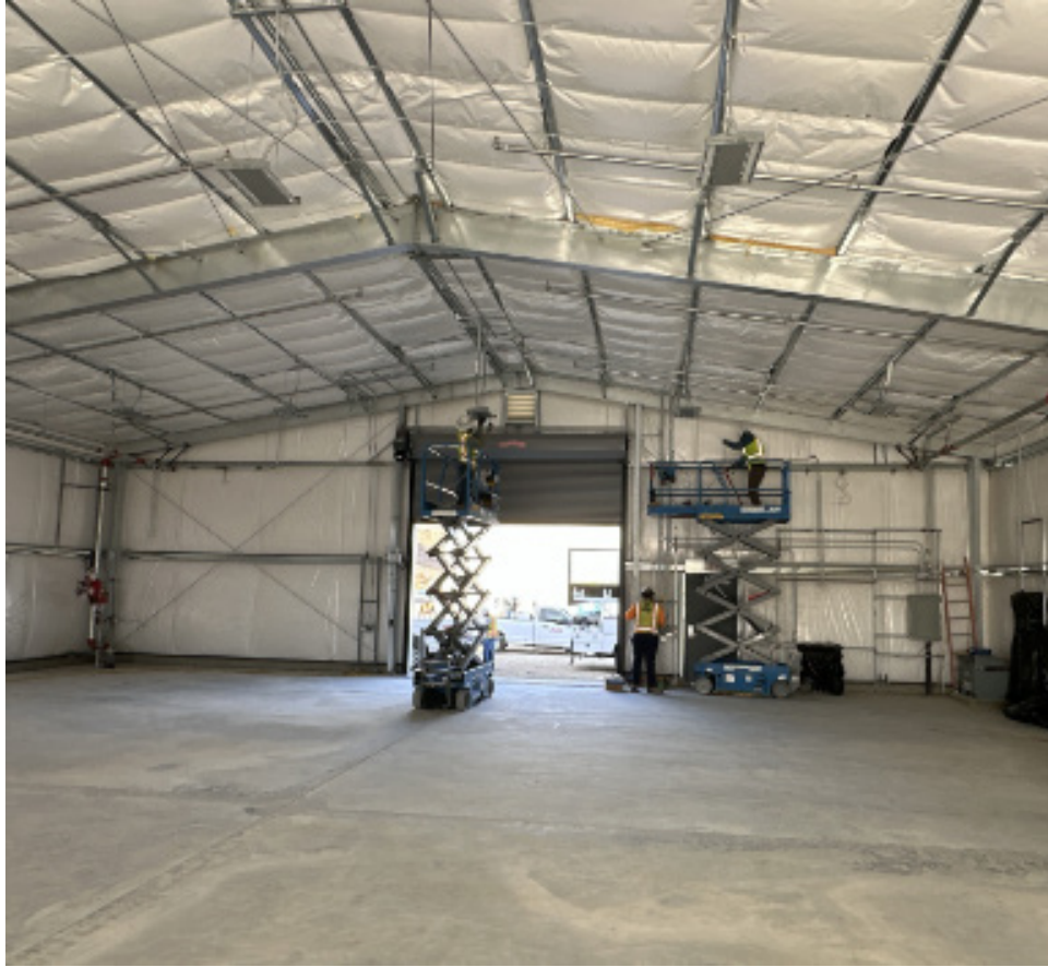
CRA Storage Buildings —Contractor Installing Conduit, Light Fixtures and Wire Pulling at the Maintenance Storage Buildings
