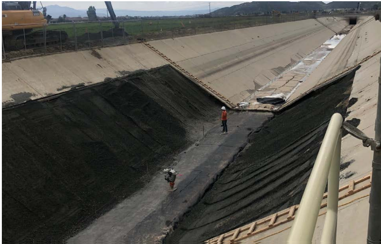
Compacting aggregate base material along side-slopes of San Diego Canal in preparation for placement of rebar and new concrete panels
