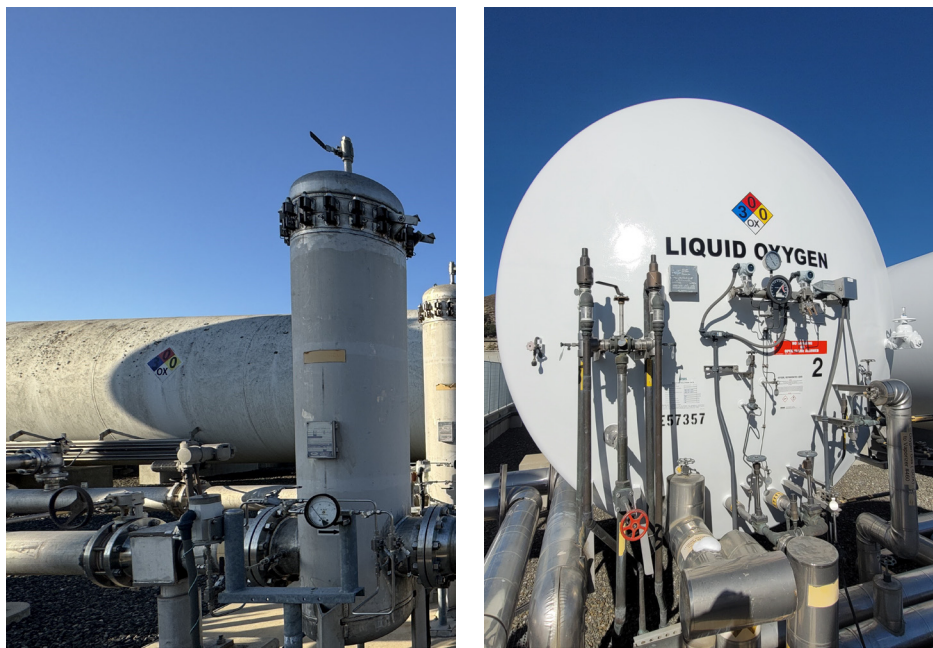
LOX tanks at the Jensen plant before (left) and after (right) refurbishment
