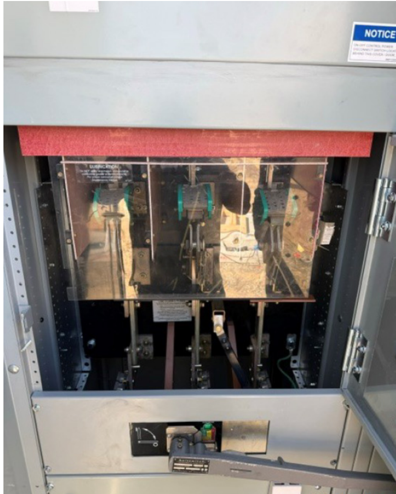
Wadsworth Bypass Pipeline – Eastside Pipeline Intertie Completed Disconnect Switch at the Southern California Edison Switchboard
