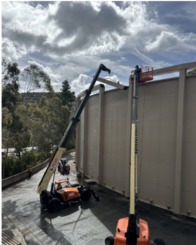
Sepulveda Feeder Pump Stations — Contractor Demolishing Box Beams on Top of Sepulveda Canyon Tank
