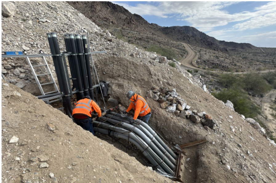
CRA Domestic Water Treatment System – Contractor Installing Reinforcing Steel at Duct Bank at Hinds
