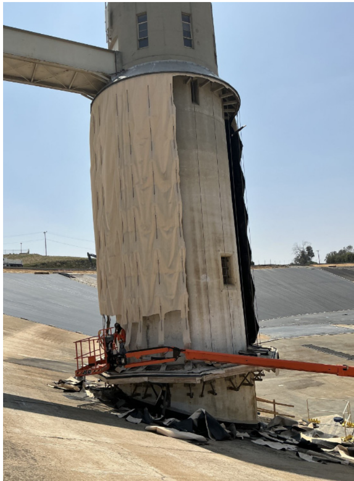
Garvey Reservoir Rehabilitation — Removing Floating Cover from the Outlet Tower Facing South
