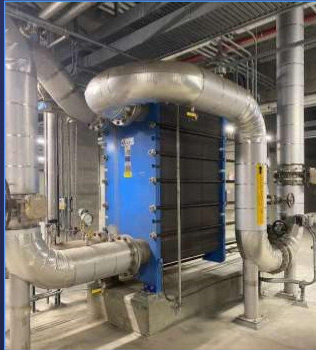
Ozone Cooling System Heat Exchanger
