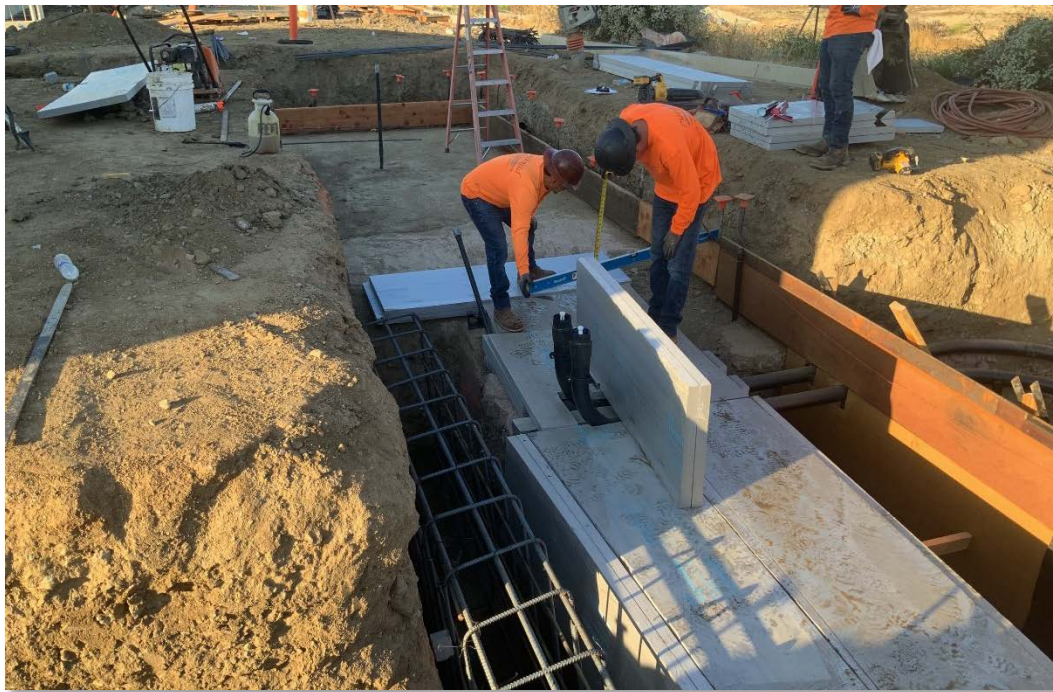
Installation of foam bond breakers for the existing electrical duct bank and reinforcing steel for the new Mills ozone switchgear building
