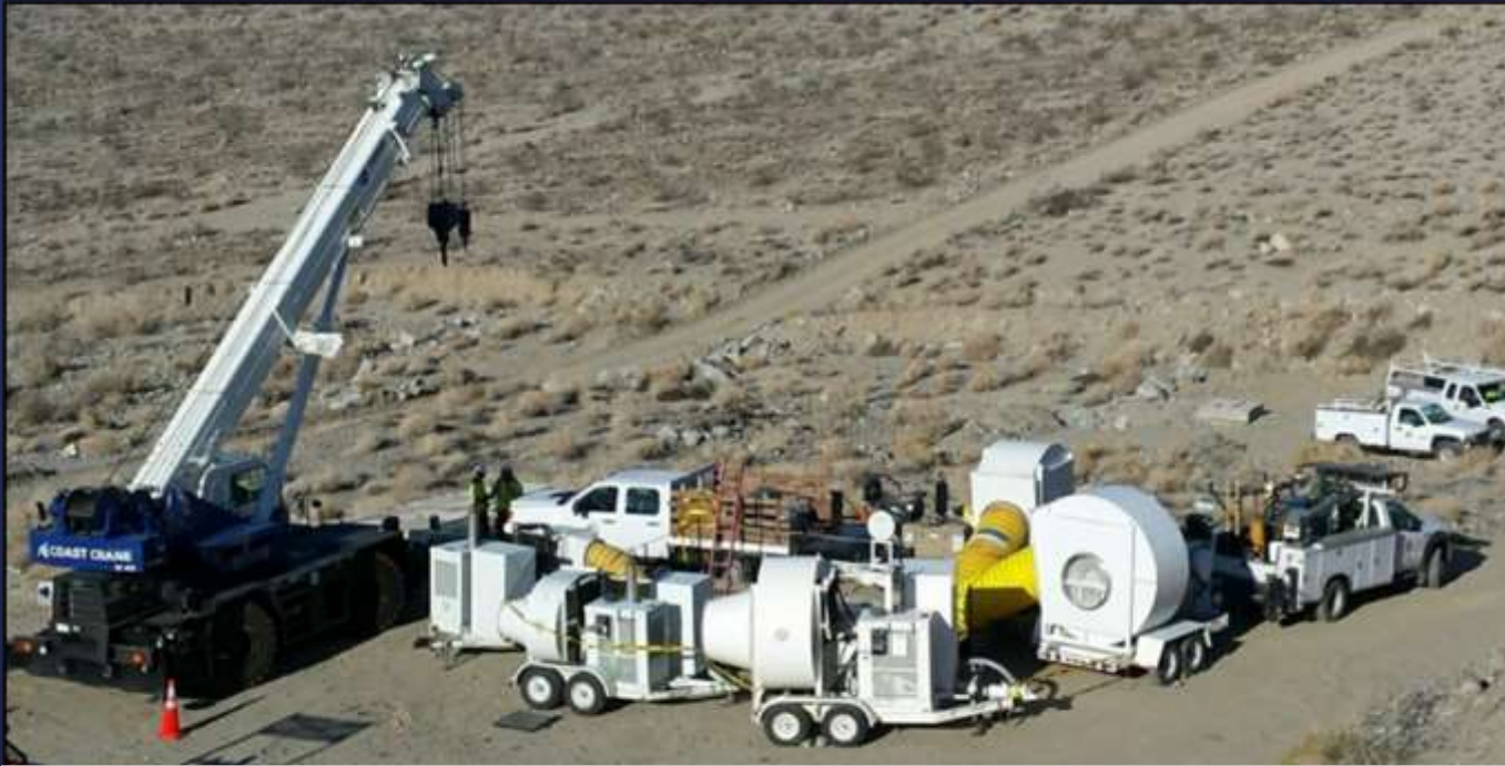
Ventillation Support Set-Up
