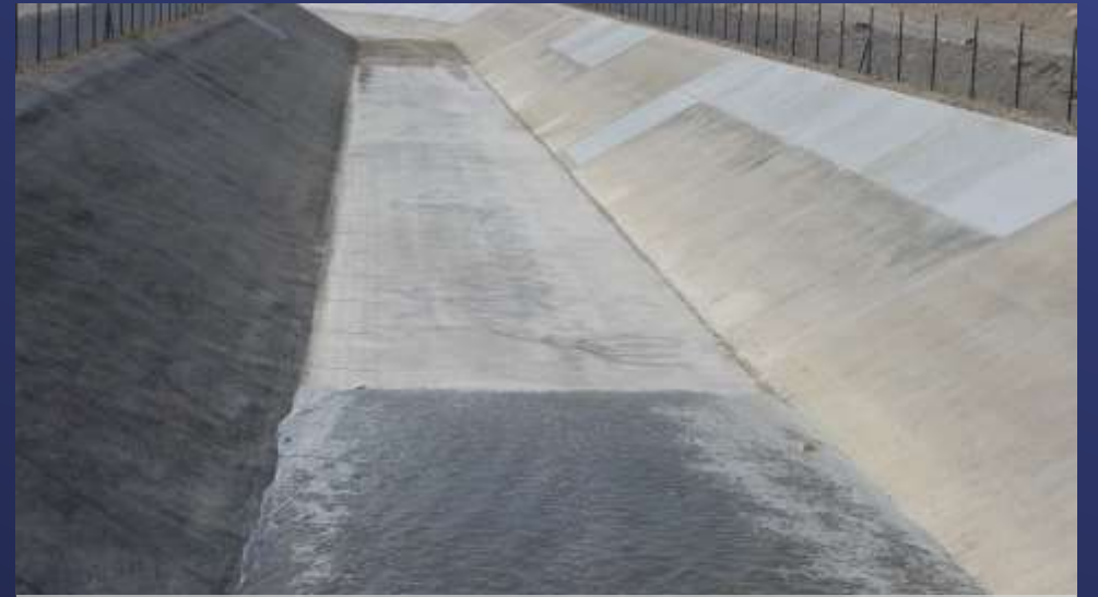
CRA Canal Flow at Start Up
