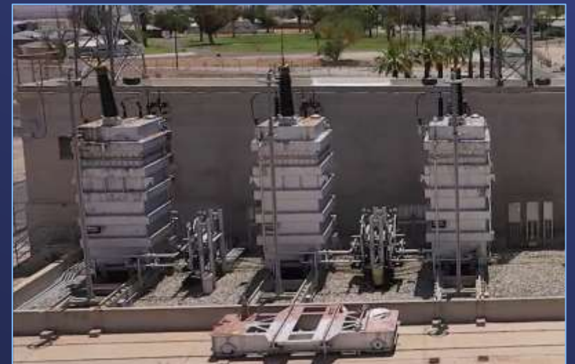
Iron Mtn. Pumping Plant
