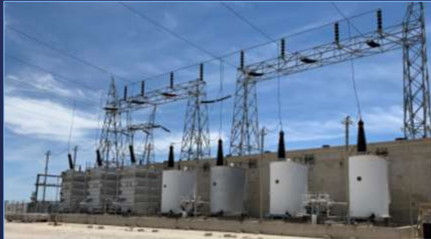
Iron Mtn. Pumping Plant
