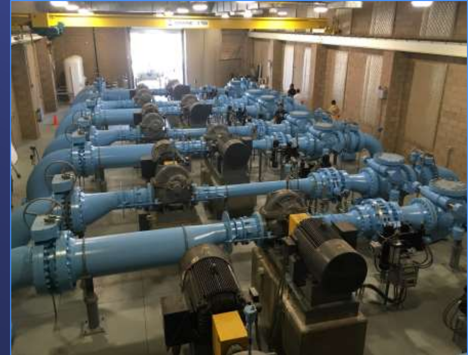
Existing Foothill Pump Station
