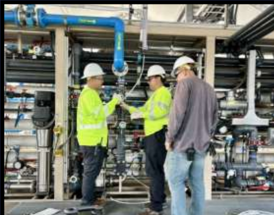
New Chemical Tubing
