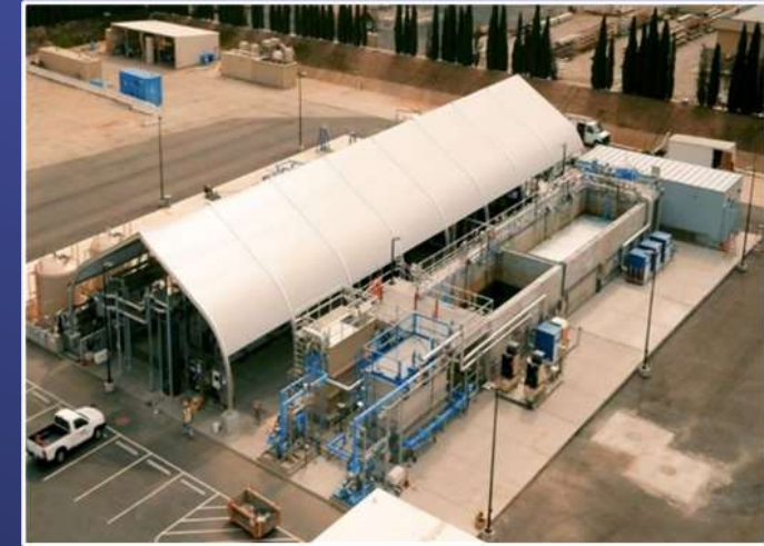
Pure Water Southern California Demonstration Plant
