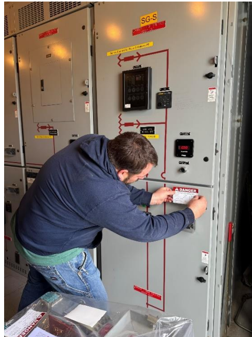
Staff adhering arc flash hazard labeling to electrical equipment at the Skinner solar facility
