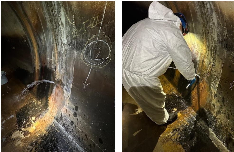
Water intrusion (left) and staff performing repairs (right) inside Rainbow Tunnel
