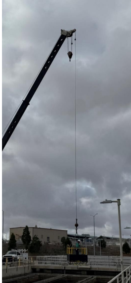
Staff working from utility basket to replace launders at Skinner washwater reclamation plant
